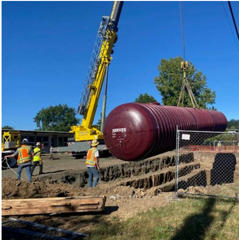
A 40,000 gallon fire water storage tank is placed at Mt. View!
