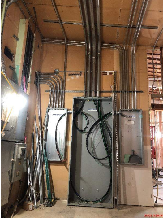
CHHS – New Electrical Room Panels
