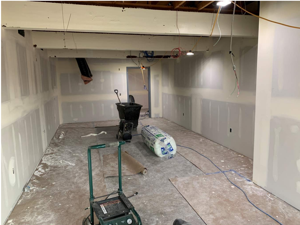
New support classrooms and offices within the center area of the existing structure
