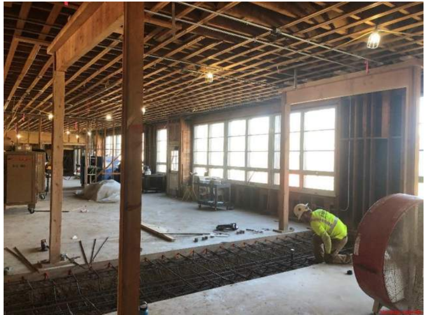
CHHS- Shear wall footing missing from original build – added new footing
