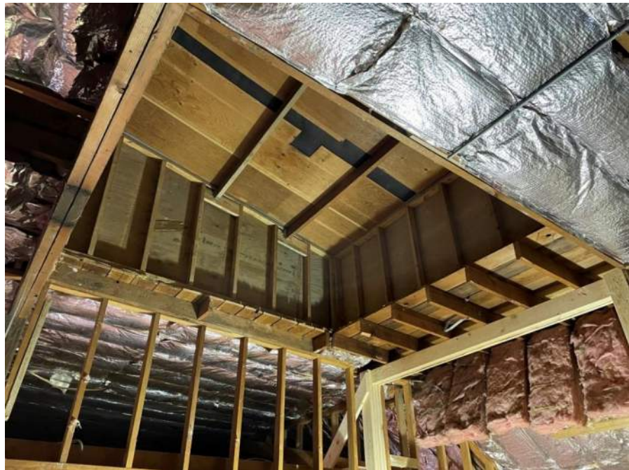
CHHS- temp roof framing to allow HVAC unit to be removed and reinstalled
