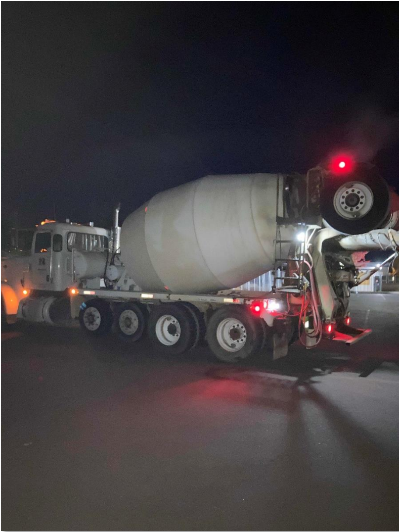
Fortis and Their Partners Working Off Hours to Accommodate the School Schedule
