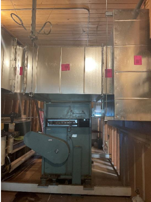
CMS – Refurbished Units and New Ductwork
