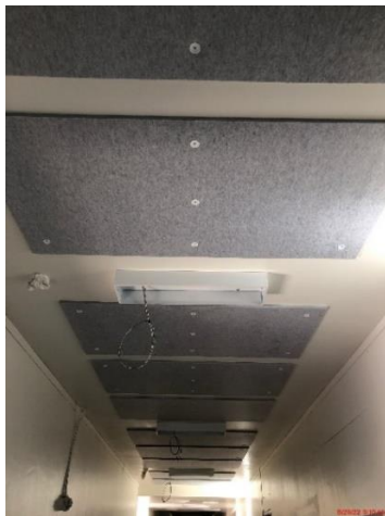
Franklin – new corridor acoustical panels
