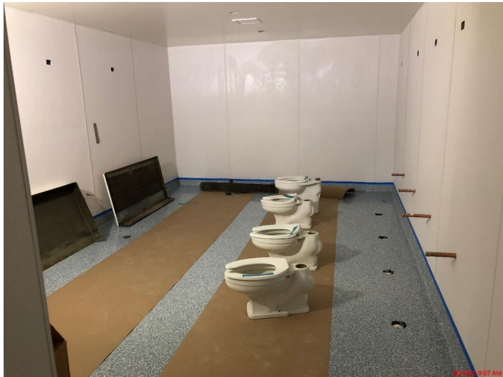
Franklin - North restroom light refresh progress, including new epoxy floors and refurbished fixtures.
