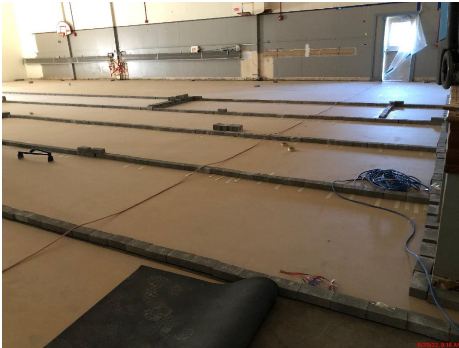
Gym Flooring in place, with protection still in place. Bricks are used to help seal the joints in the material.
