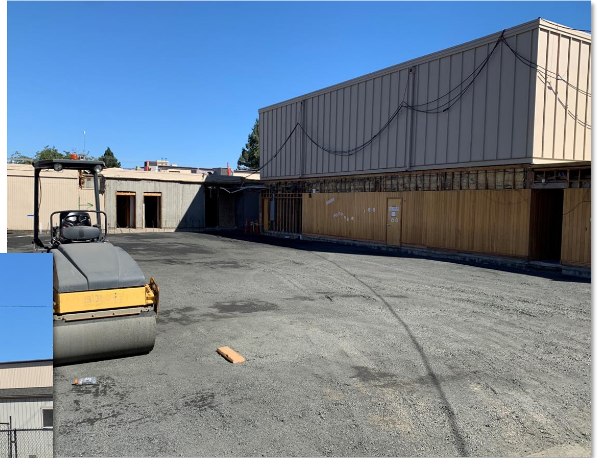
Prepping for the Art / Science Addition at the Location of the Former Locker Rooms
