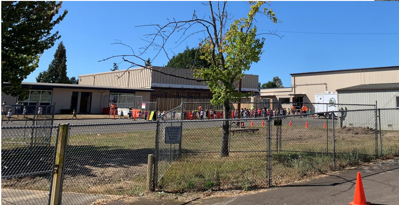
Temporary office on the Right with New Office Construction in the Background. Kids are Using the Temporary Routing Around the Construction Zone
