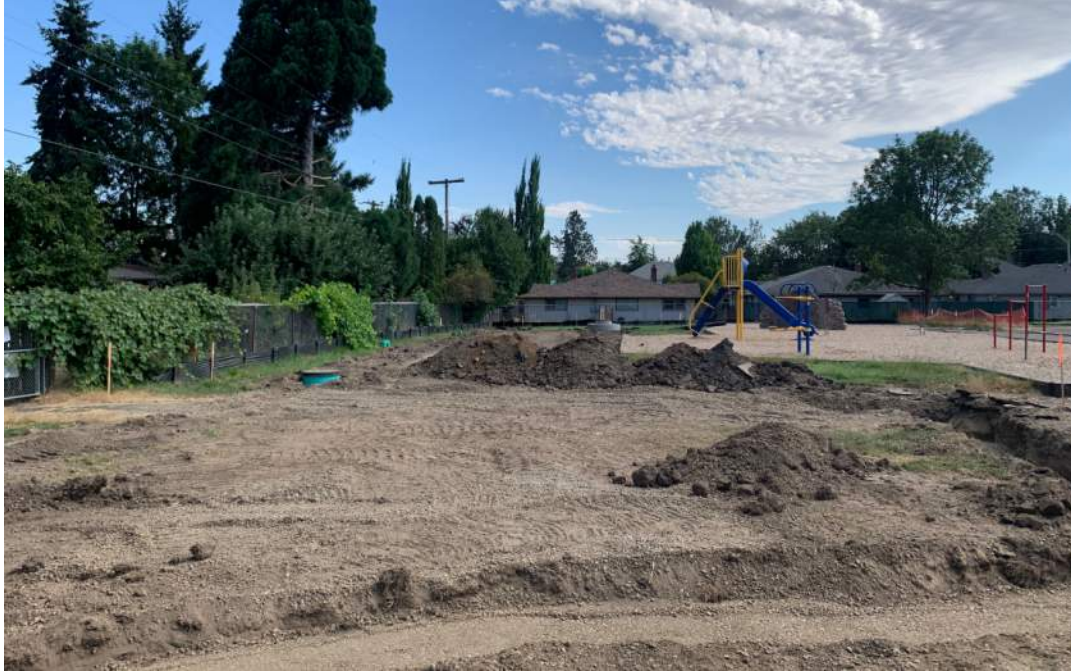
Storm detention system
