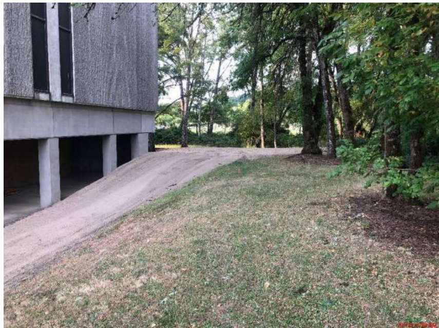
Bldg. A – Crane Ramp for structural work (will be removed in August)
