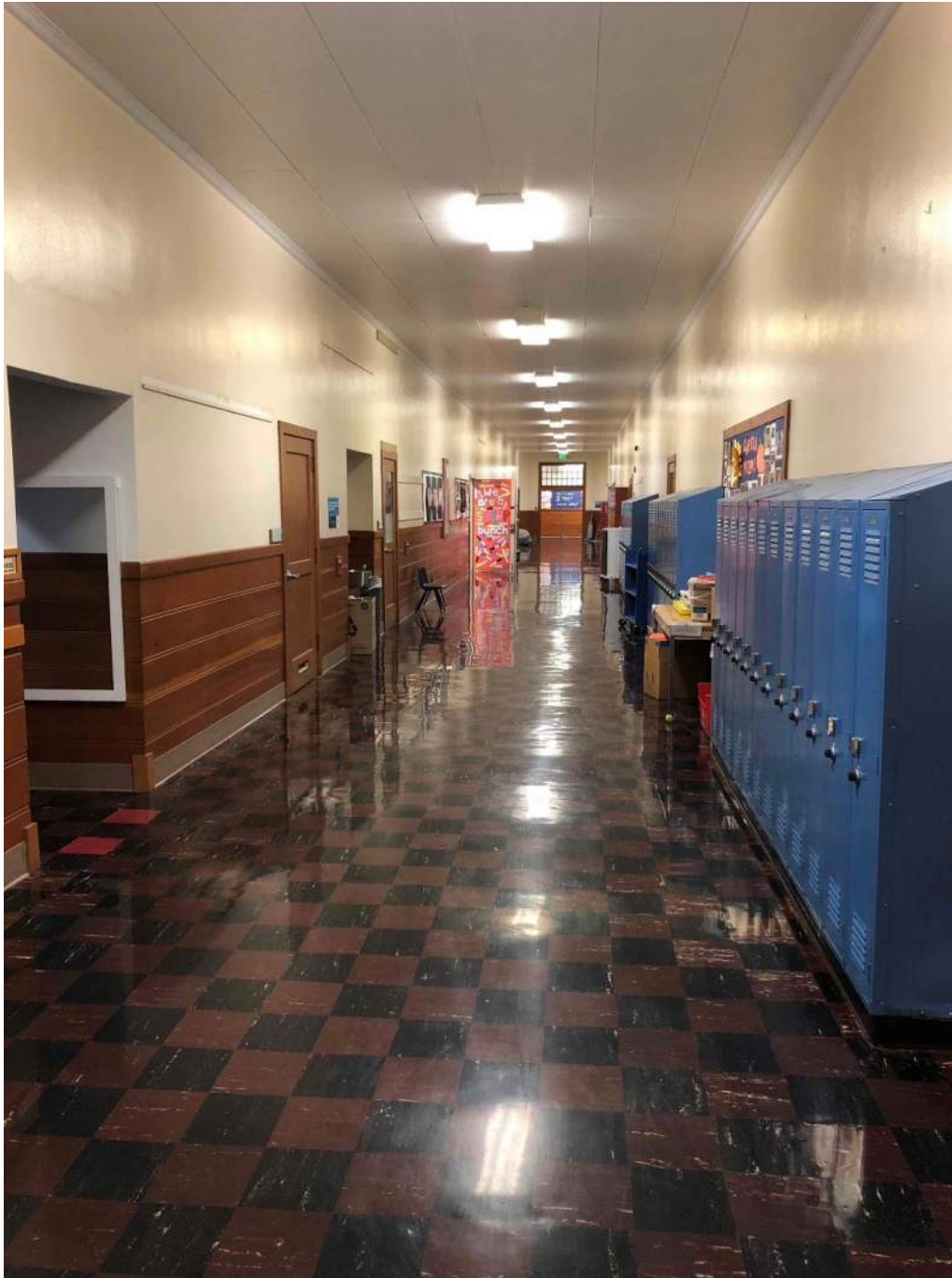
Franklin Hallway - flooring to be abated
