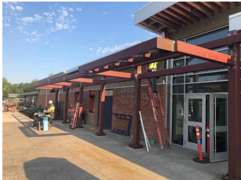
GES – Front Entry canopy progress – see through solar panels will be installed here
