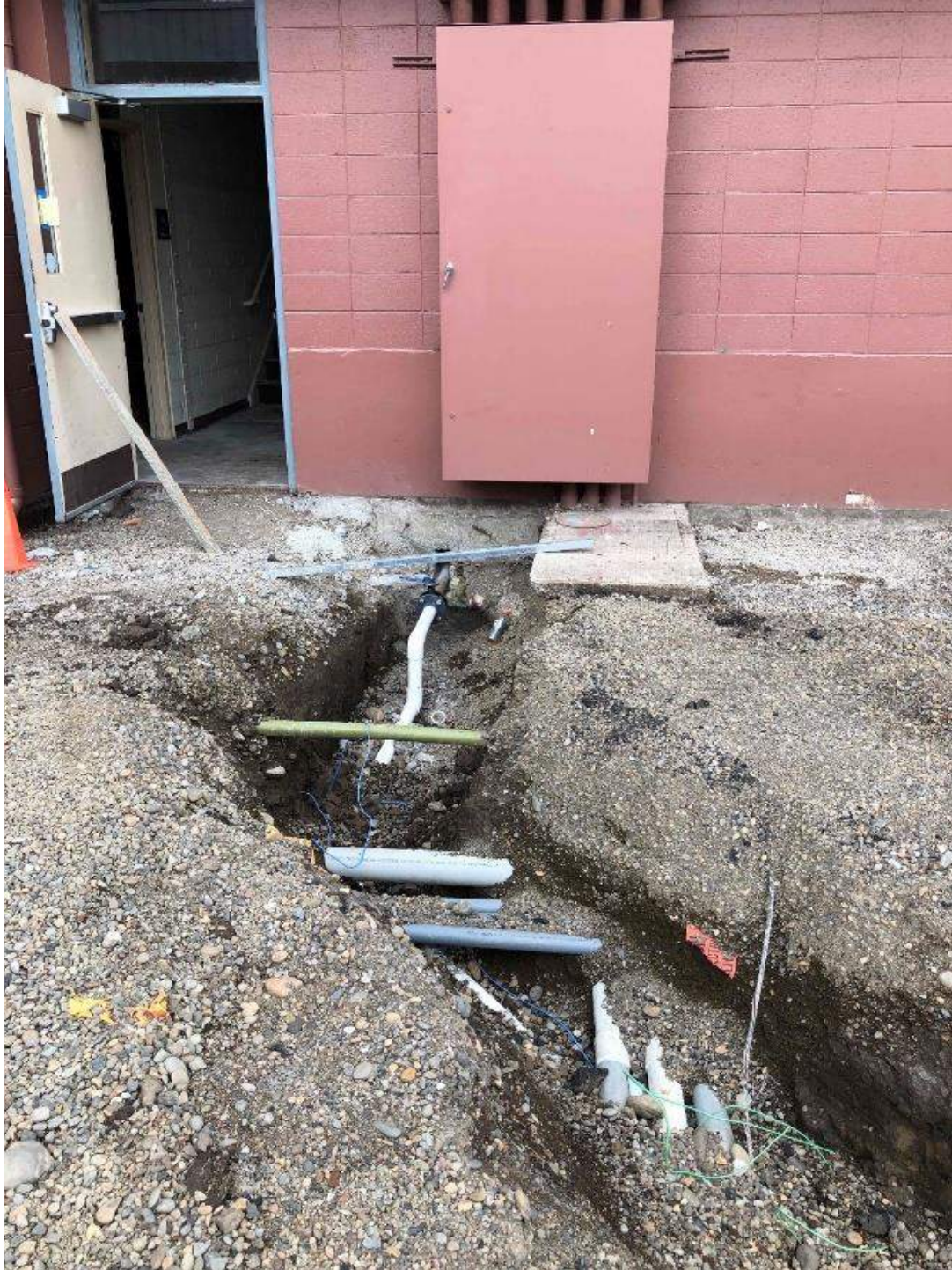
CHS - underground obstacles
