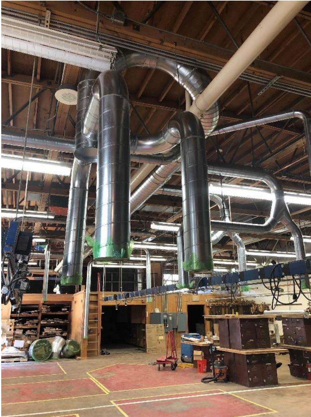
CHS – new woods dust collector piping
