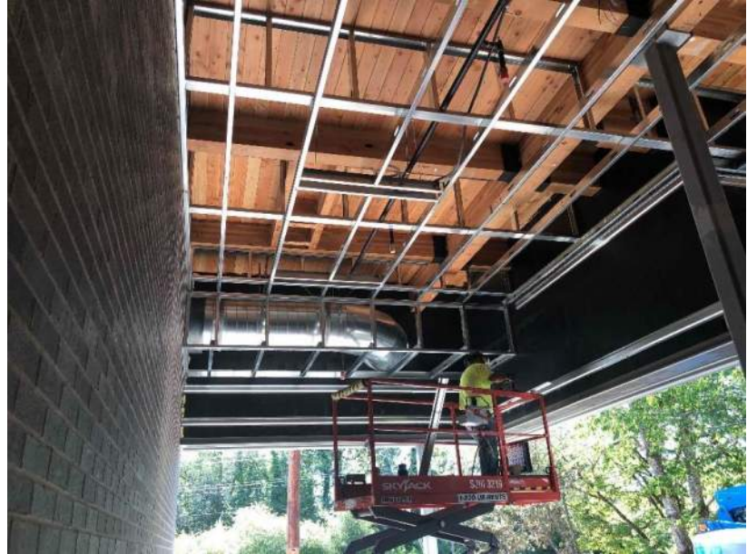
CVHS Building F – metal ceiling ready to begin at outdoor kiln area
