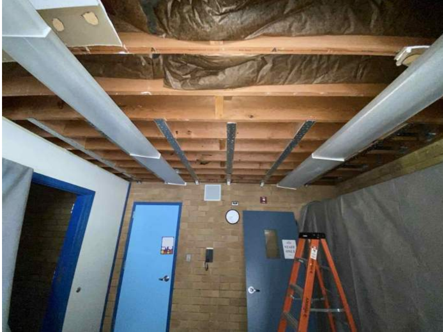
CMS seismic work installing in ancillary rooms on N & S ends of Library
