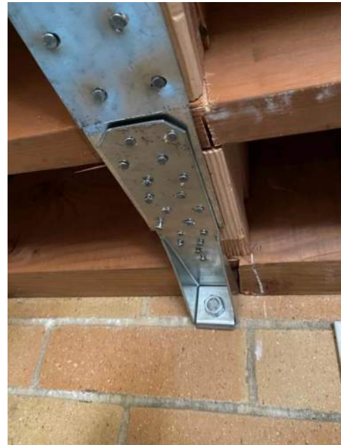
Library seismic strapping
