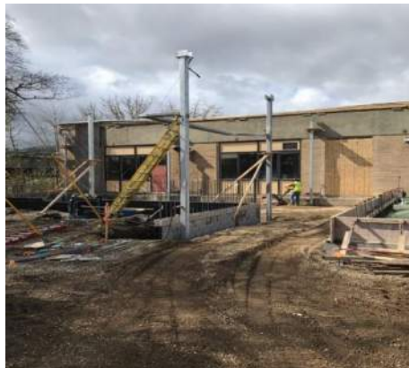
CVHS Outdoor work area – foundation walls up (left side) and new building footprint
