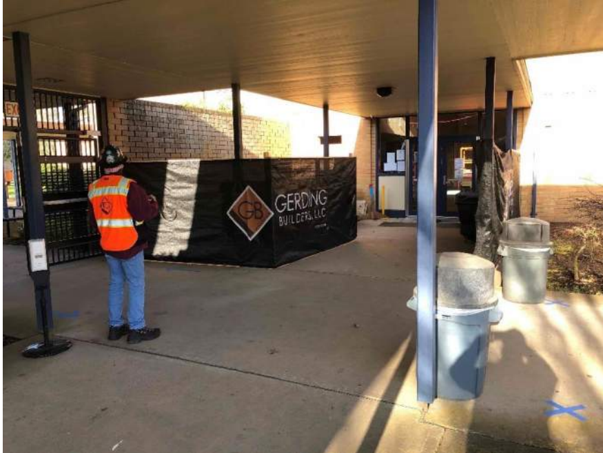
A Gerding devised movable gate to keep students and const workers separate
