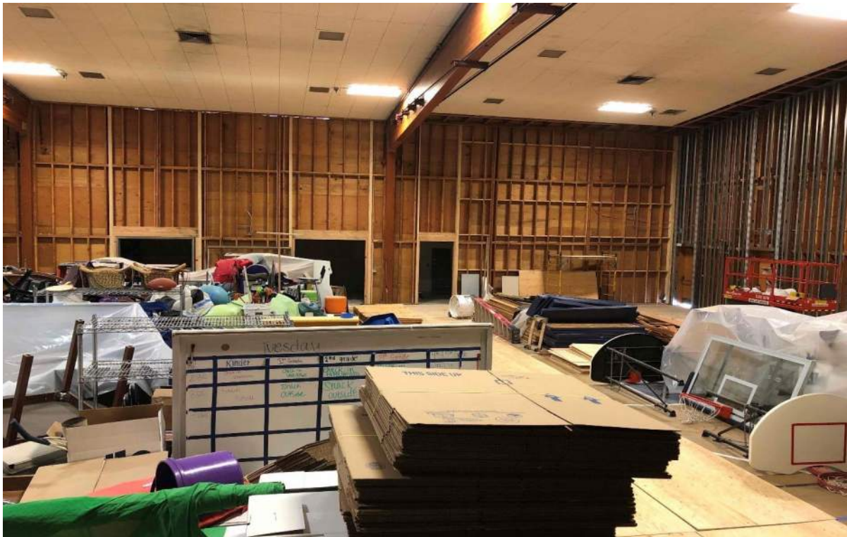
Gym strongback wall work on right and new openings for PE office and storage
