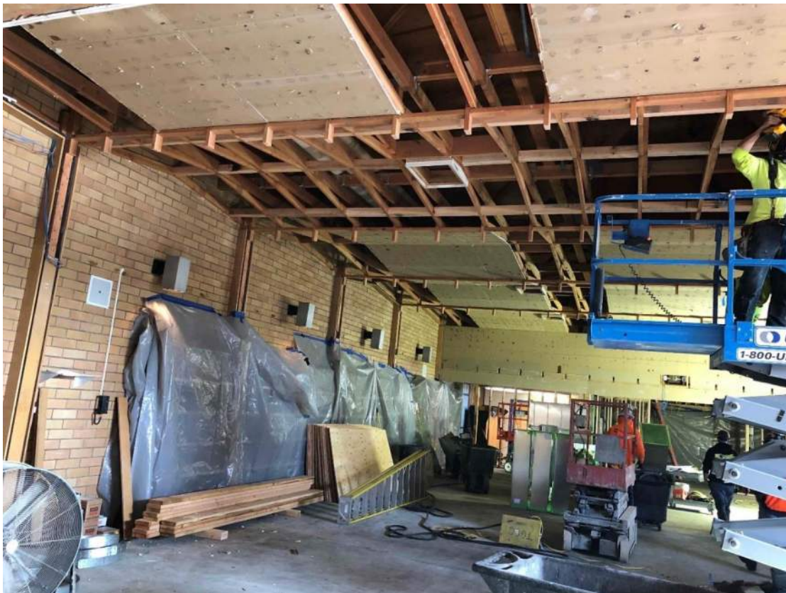
Library ceilings removed in order to remove old duct and to install new ceilings & lighting
