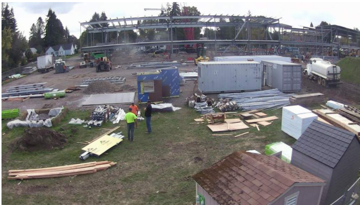
A webcam view of the LES site, dated 10/12/2020 showing the steel framing
