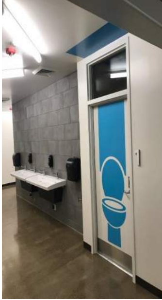
Cheldelin Individual Restroom & sink
