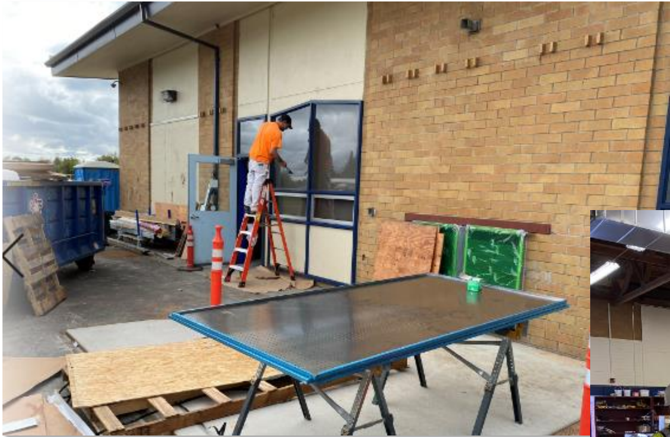
Cheldelin mat room exterior and interior with Paul Jennison showing the much-needed HVAC improvements
