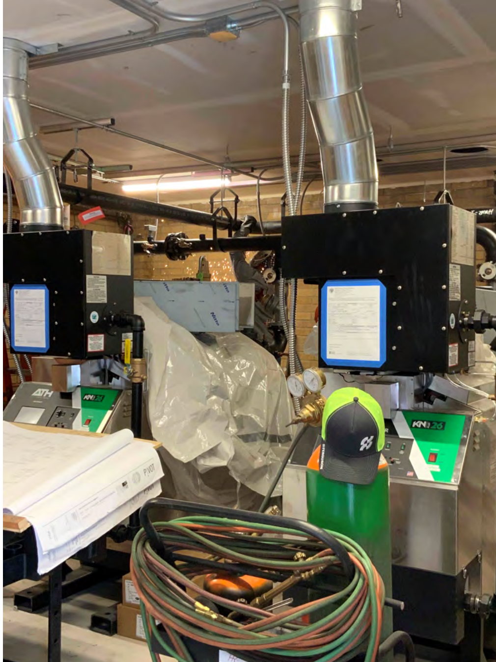
New Boilers are installed and have been fired
