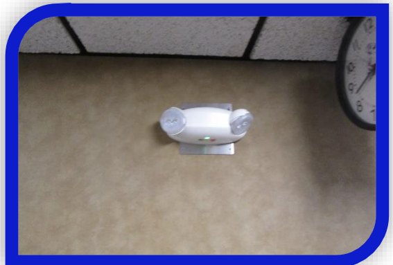
Emergency Lighting System
