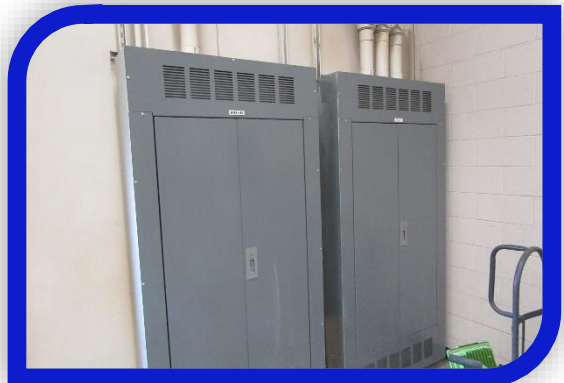
Main Electrical Distribution System
