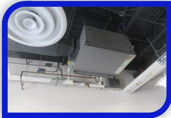
HVAC Terminal Unit
