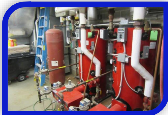
Hot Water Boilers
