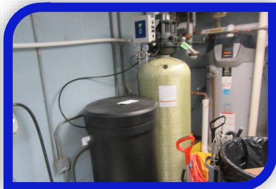
Water Softener System
