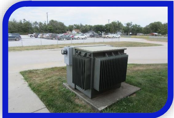
1 of 2 Transformers Serving Building
