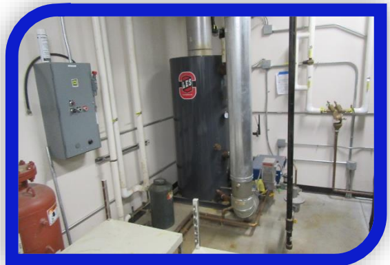
Hot Water Boiler
