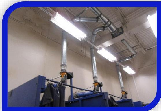
Welding Ventilation System
