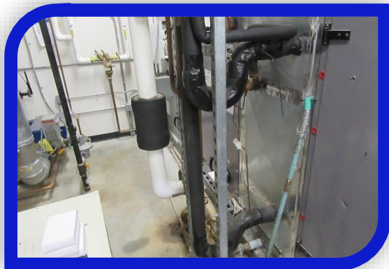
Air Handling Unit #1
