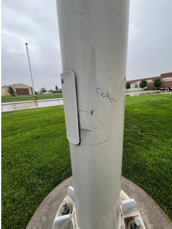
Cracked light pole at handhole
