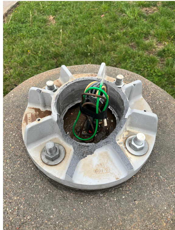
Failed light pole base casting
