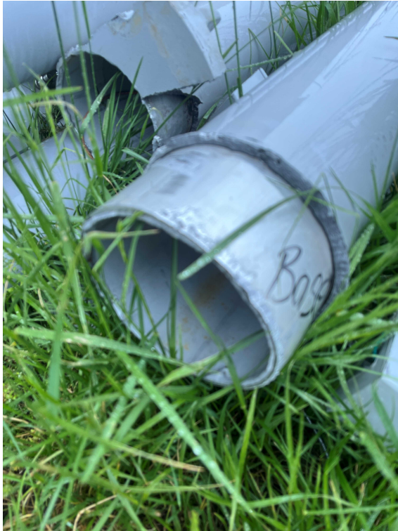
Failed light pole base
