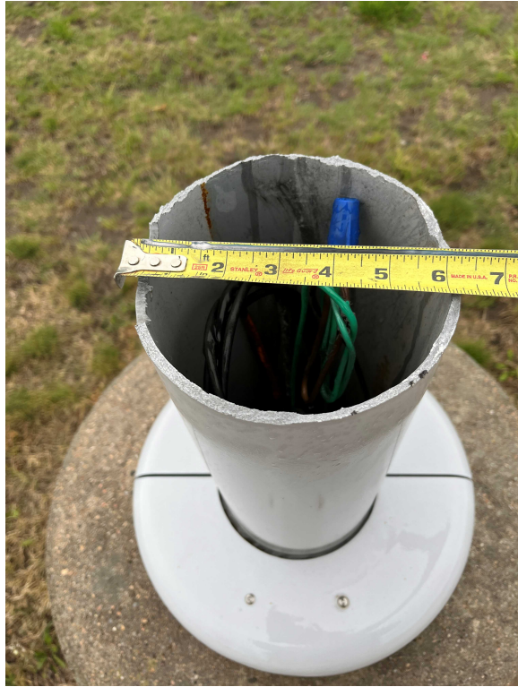
Failed light pole at handhole
