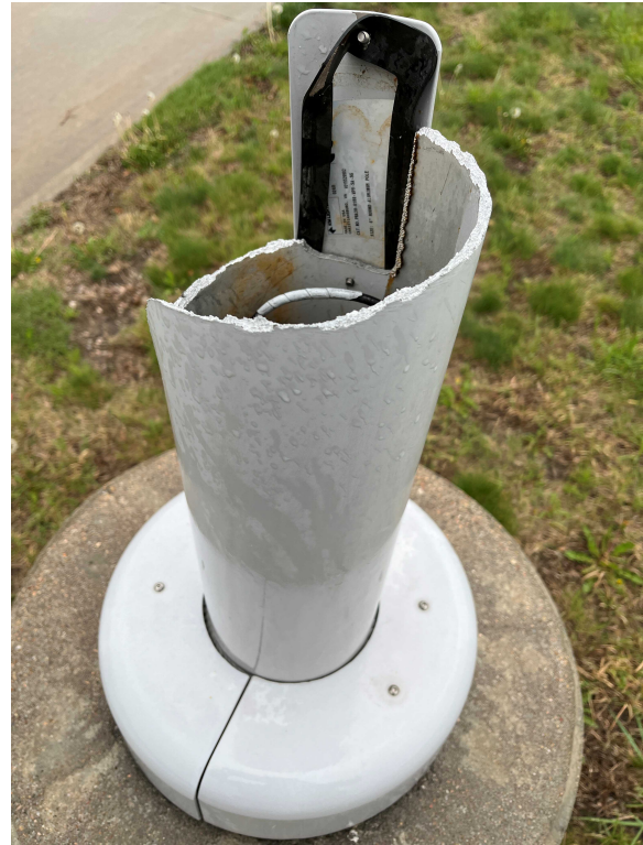
Failed light pole at handhole
