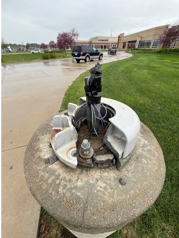
Failed light pole base casting
