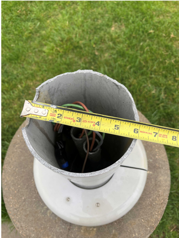
Failed light pole at handhole
