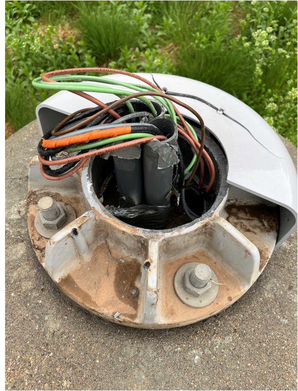
Failed light pole base casting
