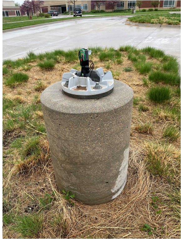
Failed light pole base casting
