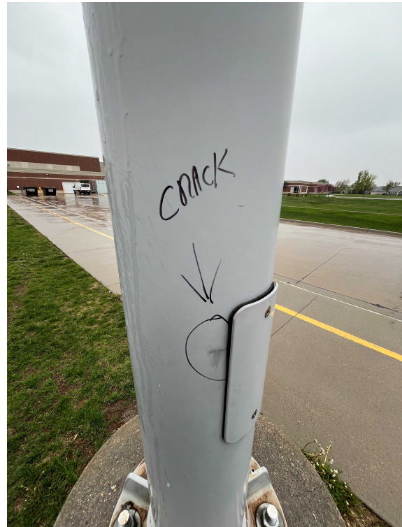
Cracked light pole at handhole
