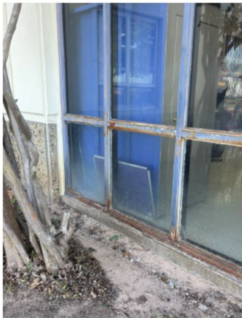
Deteriorating exterior finish
