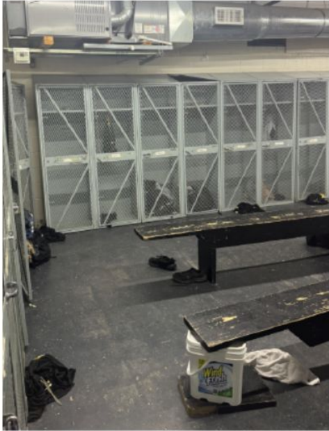
Deteriorating finishes at the Field House at Junior High
