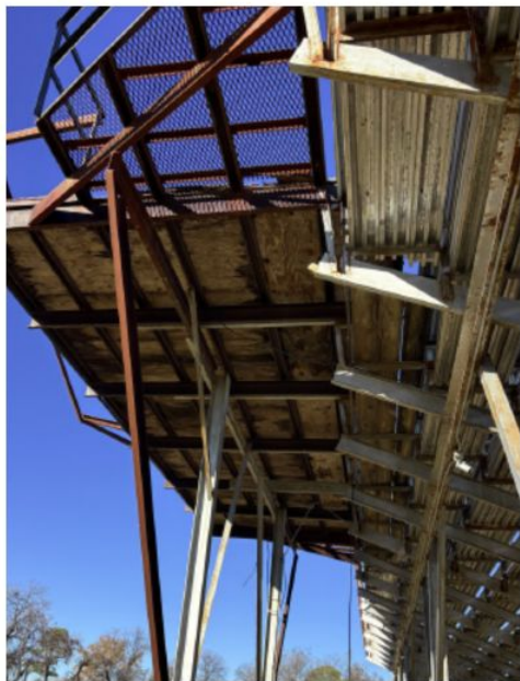
Evidence of rust at the bleachers at Junior High Football Field
