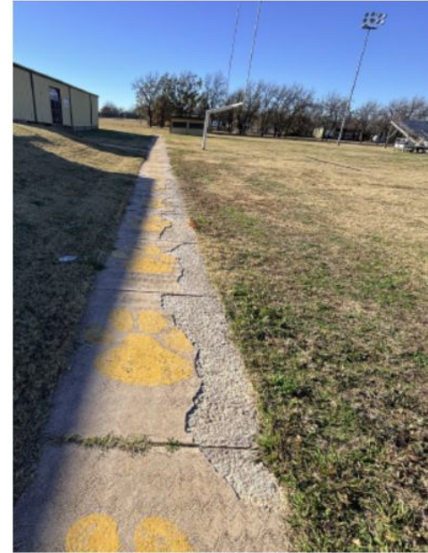
Sidewalk cracking and damage at the Field House at Junior High School
