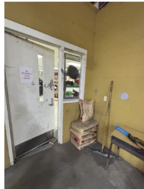
Deteriorating door finish
