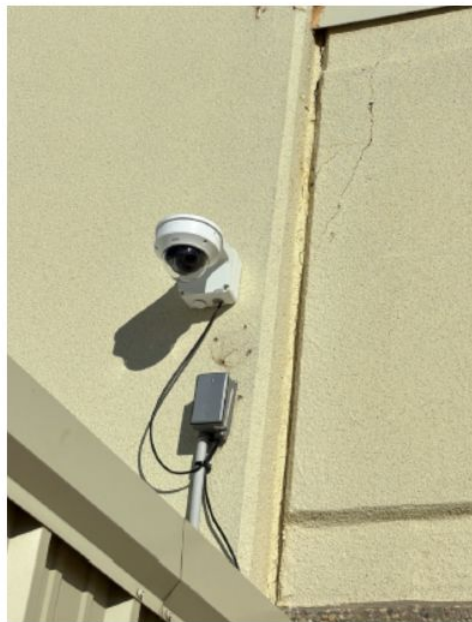
Evidence of cracking at building joint
