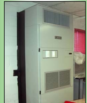
New Energy Efficient HVAC Equipment
