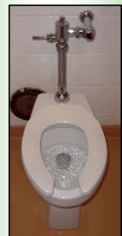
Domestic Water Replacements [Low-Flow Toilets]
