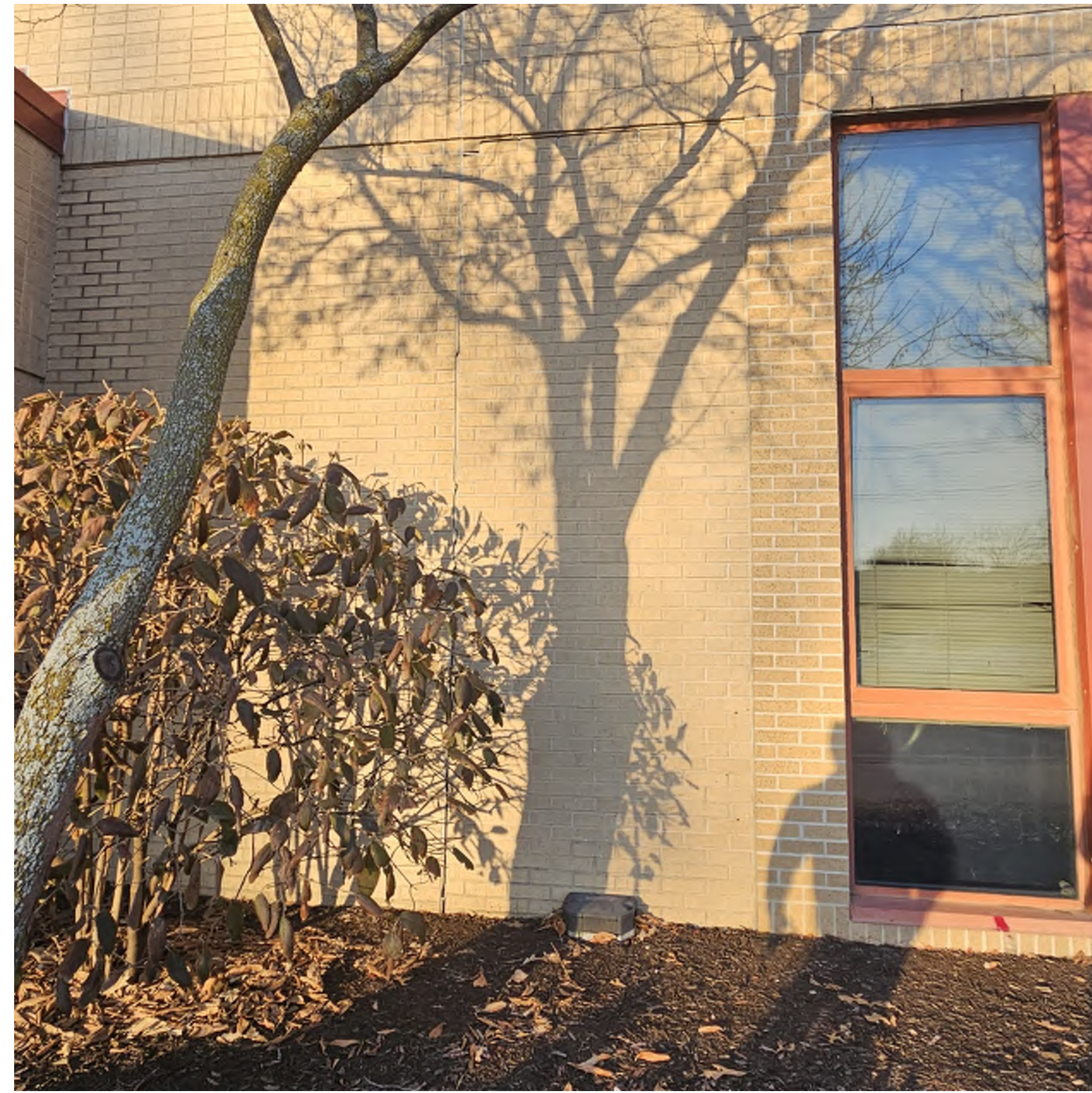
2 G110 EXISTING CRACKED BRICK/JOINTS
