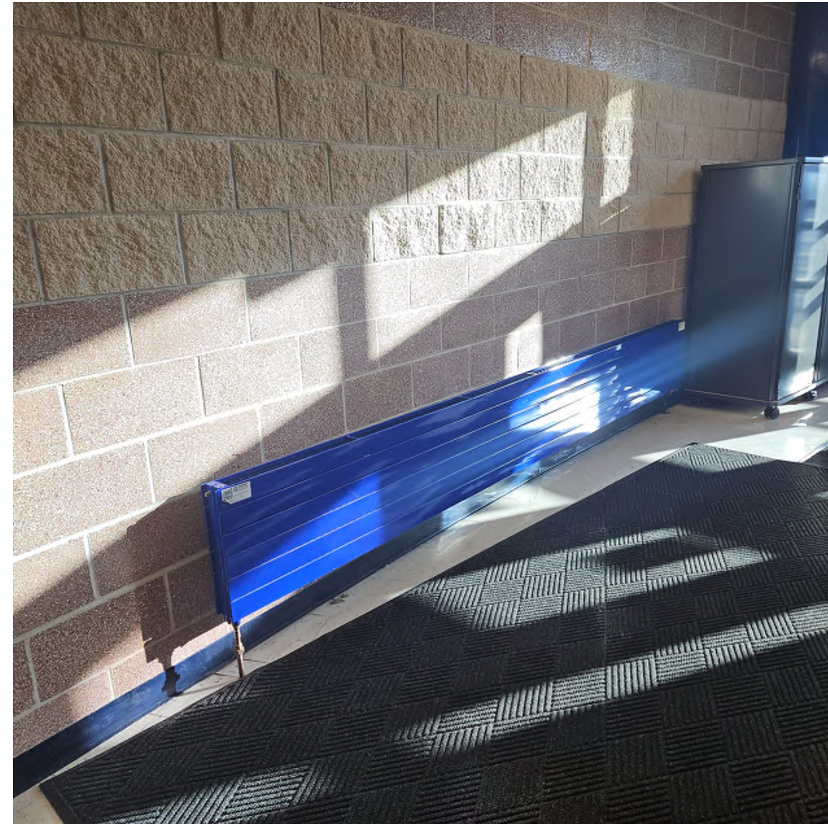
2 G125 EXISTING HVAC WALL UNIT
