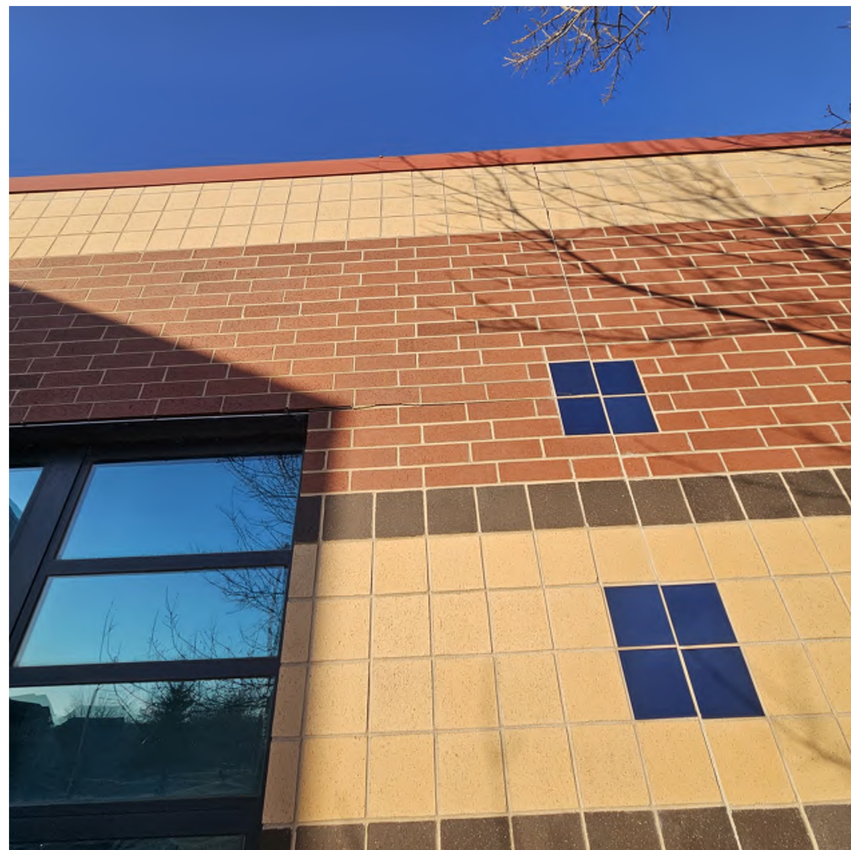
4 EXISTING CRACKED MASONRY JOINTS G120
