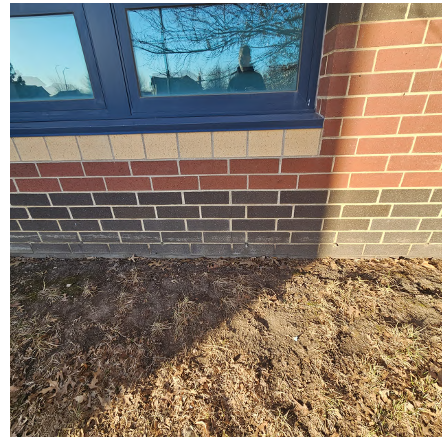
3 CRACKED BRICK/JOINTS BELOW WINDOW G120
