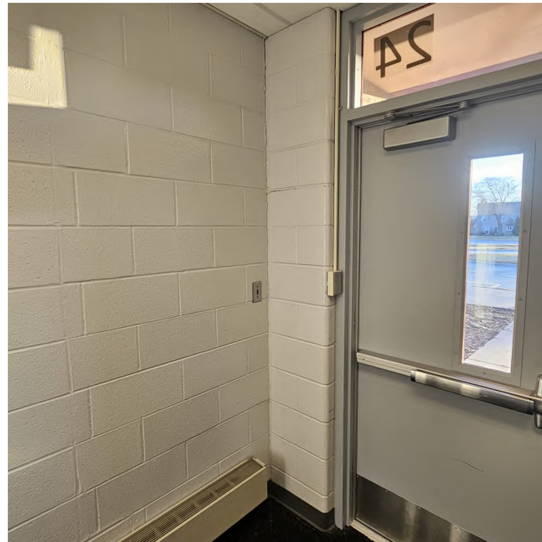
5 G110 EXISTING CRACKED JOINTS
