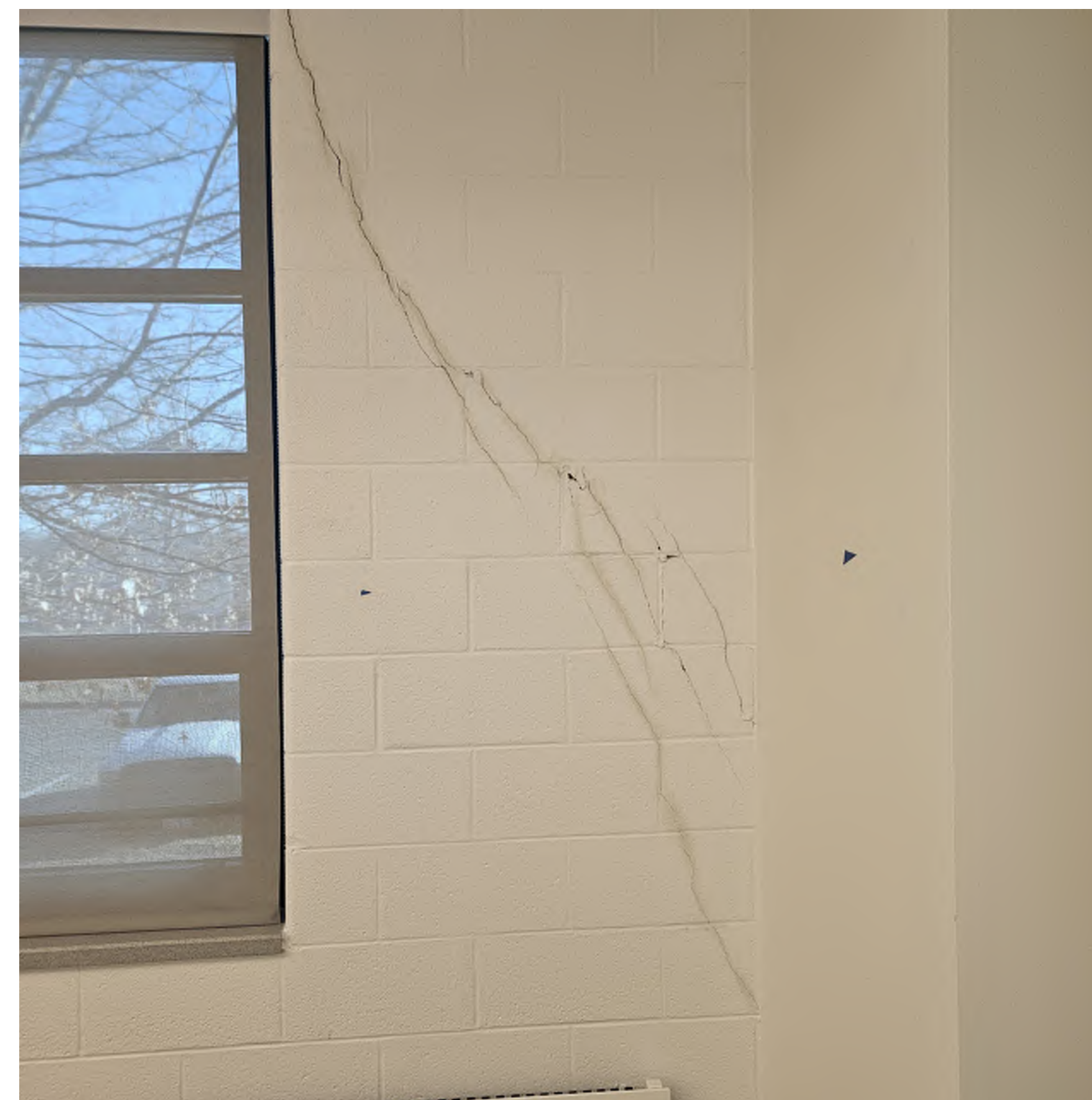
5 G125 EXISTING CRACKED CMU
