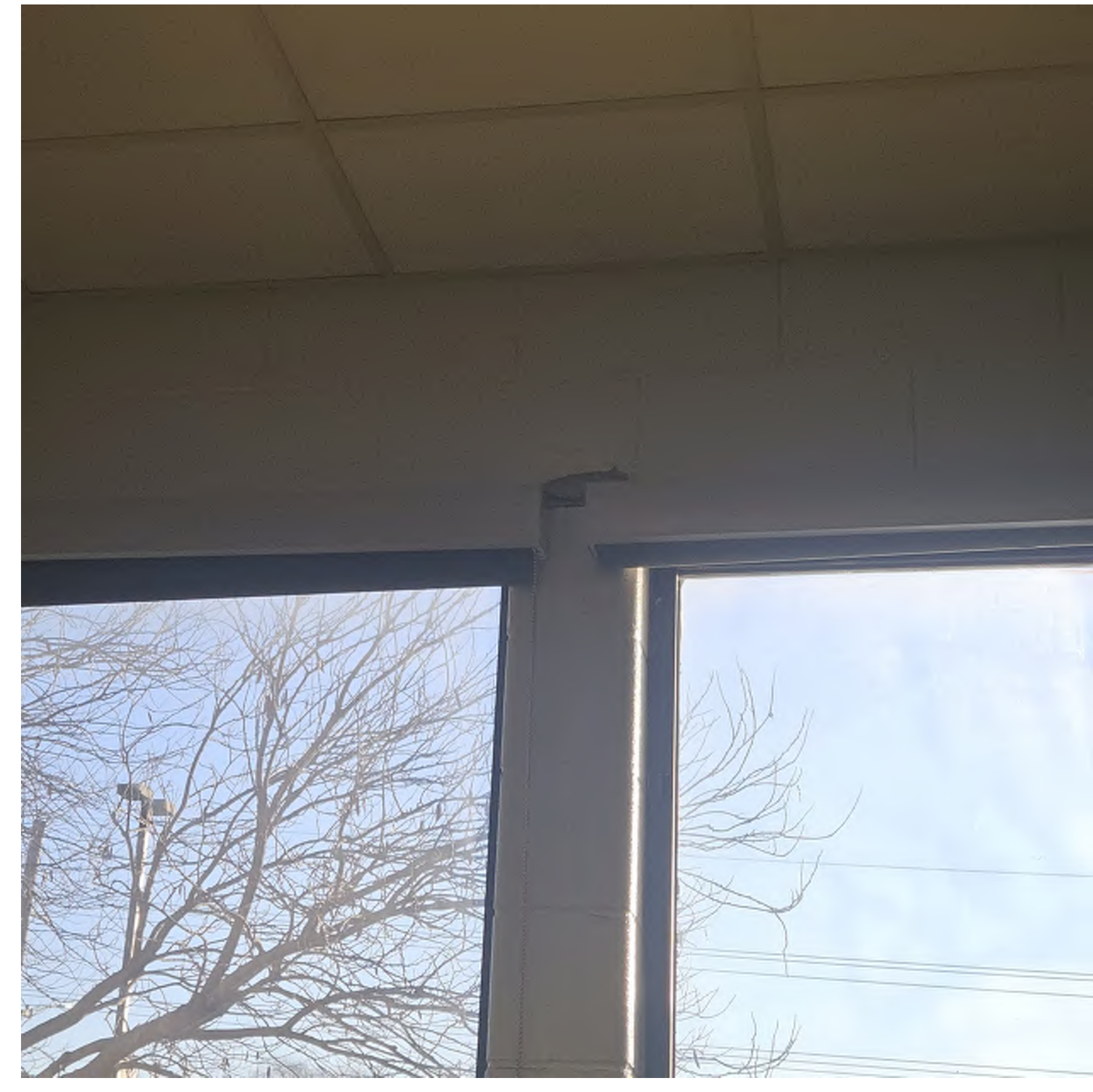
3 G111 CRACKED ABOVE CMU WINDOW
