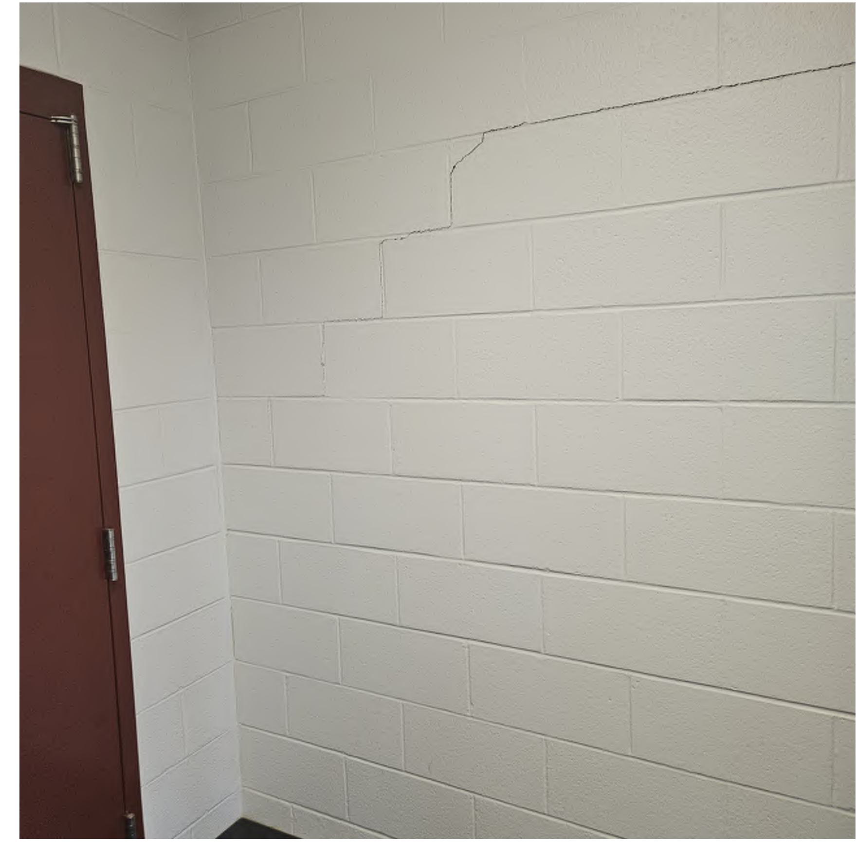
3 G100 EXISTING CRACKED MASONRY
