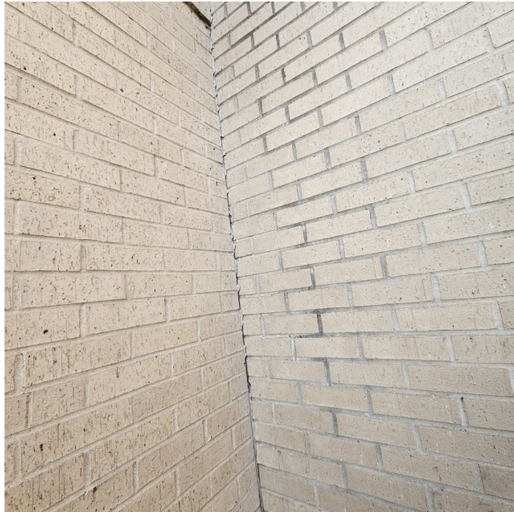
1 G110 EXISTING CORNER CRACKED JOINT
