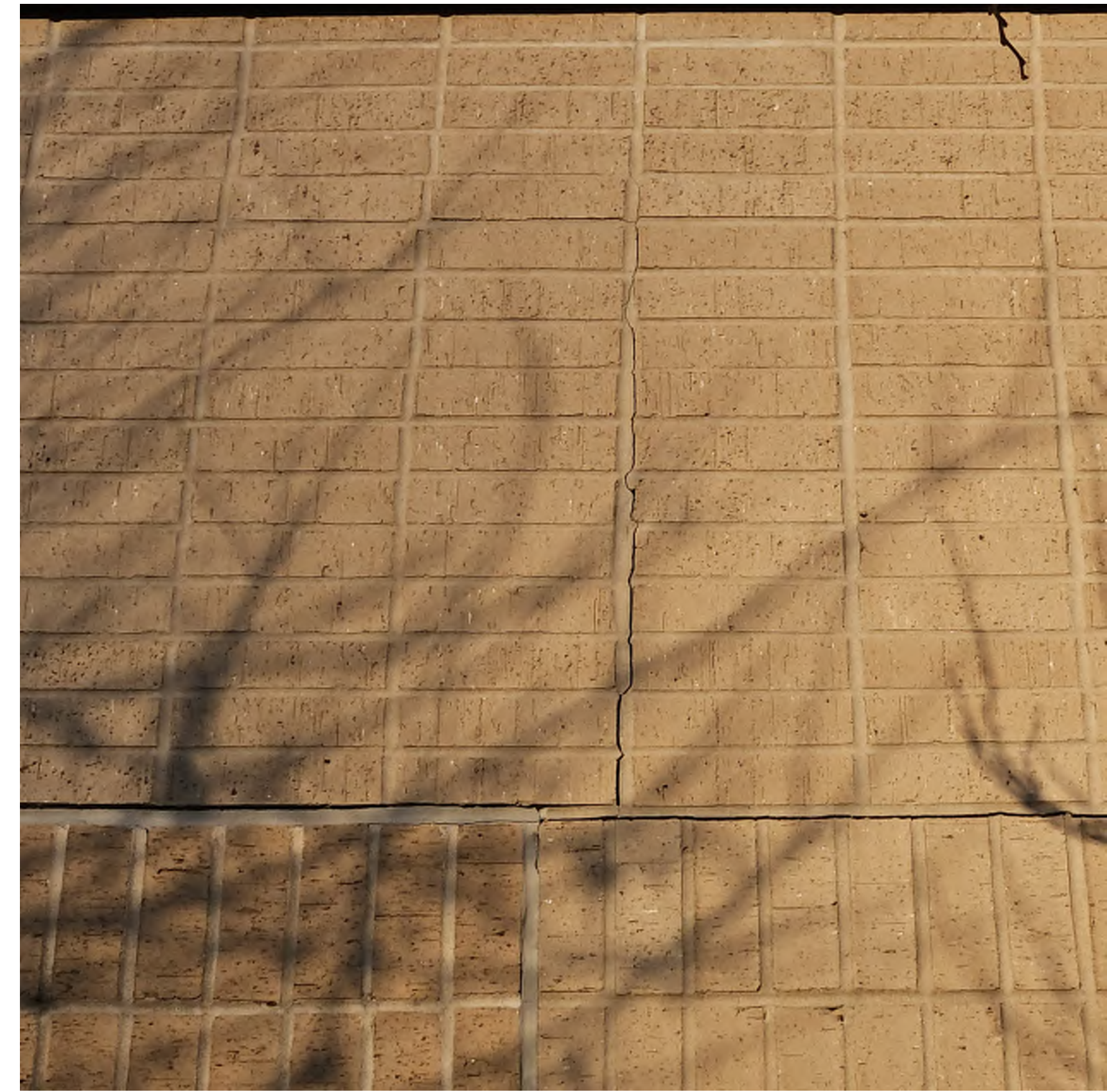
3 G110 CRACKED JOINTS ABOVE WINDOW
