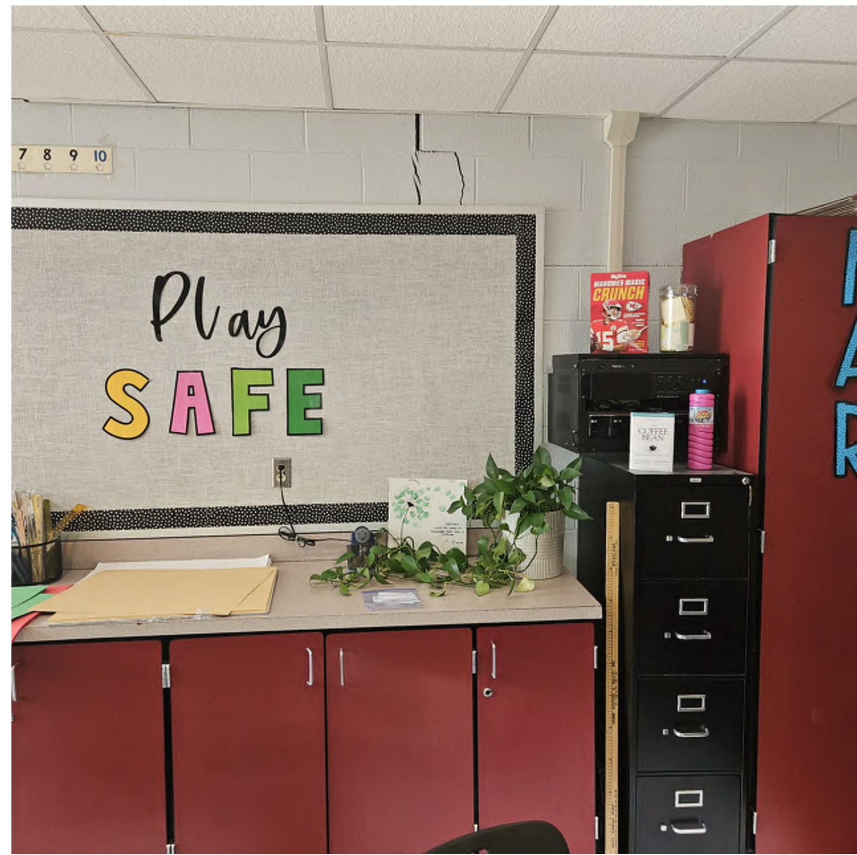
5 G100 EXISTING CRACKED CMU / TACKBOARD
