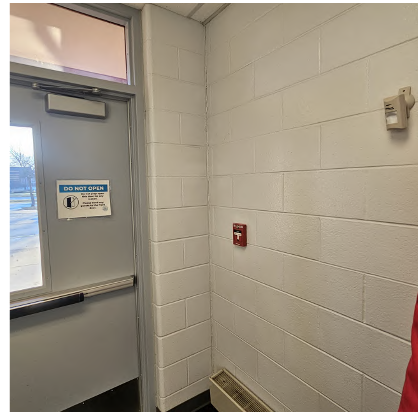
6 G110 EXISTING CRACKED JOINTS
