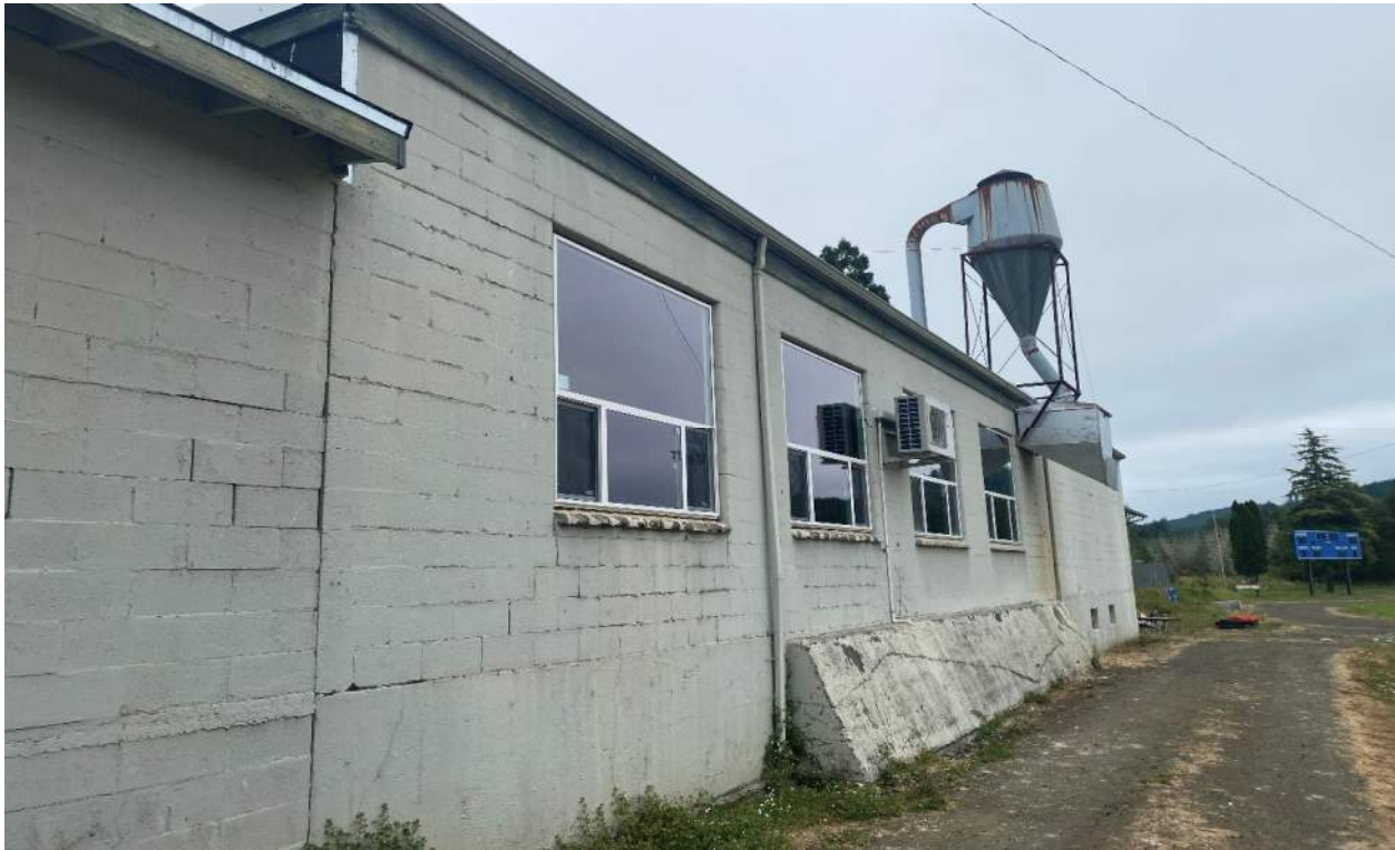
Photo 5: North Wing – Wood Shop – CMU Wall – Attempted Exterior Repair – Wall Physically Flexes with little effort of pushing. Inadequate supported mechanical equipment.
