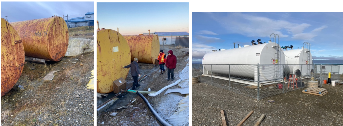
TLA Fuel Storage tanks, Planning, New tank farm
