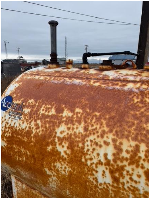
Teller new bulk fuel facility. tanks.
