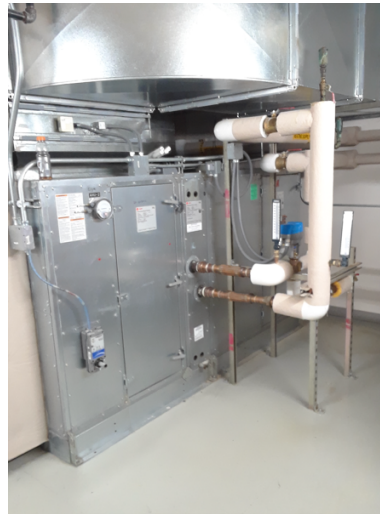
714 715 A newer up to date HVAC unit
