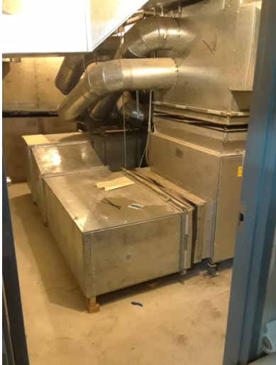
712 713 An older HVAC clunker.
