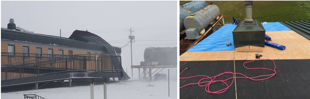
Wales school roof damage and repair 2017. Now the rest of the roof is threatening to fail
