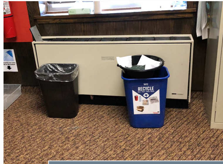
YMCA Room PTAC style units have had ongoing maintenance issues and should be considered for replacement
