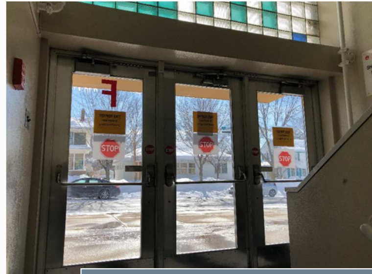
Multiple older exterior doors throughout facility with inefficient single pane glass
