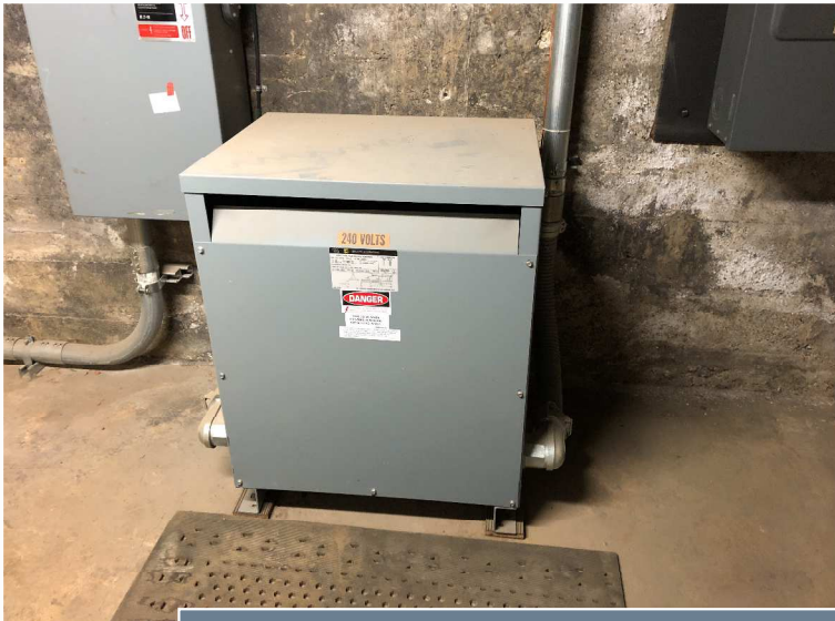
Electrical service is not sized for building dehumidification
