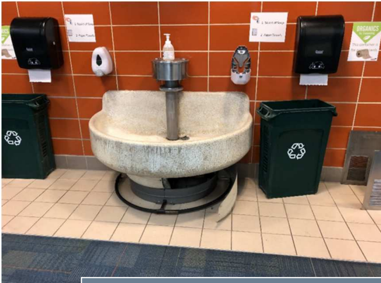
The 1970 restroom wash stations have been a maintenance issue and should be replaced
