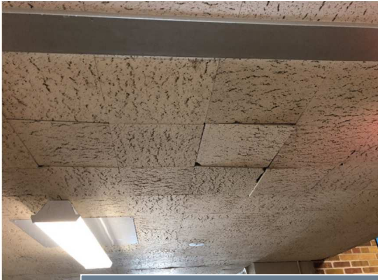
Original adhered ceilings in need of replacement
