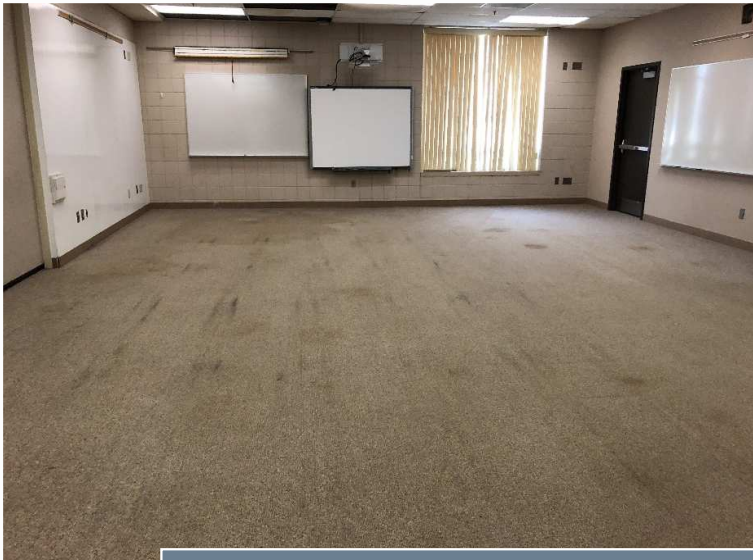
The rolled carpet flooring throughout much of the facility is from 1994 and is well beyond its expected service life
