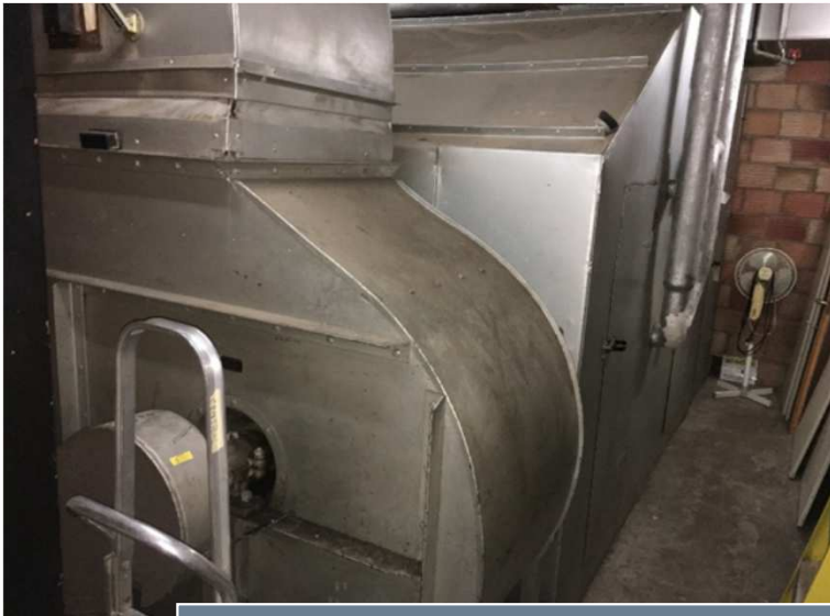
Multiple central ventilation systems are original and over 70 years old
