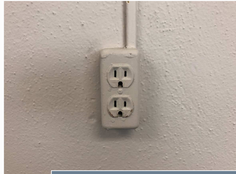
Most of the electrical distribution is beyond it's expected service life and may not meet 21 st century education needs
