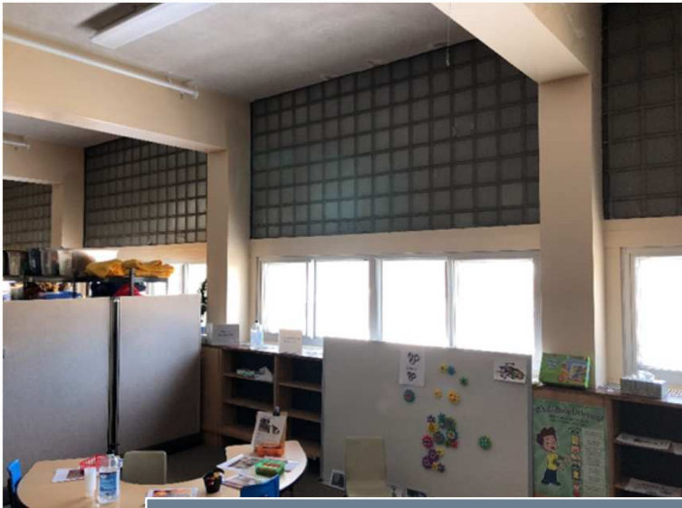
Some older inefficient windows throughout facility – STEAM room windows leak when it rains. Glass block is cracked in many areas
