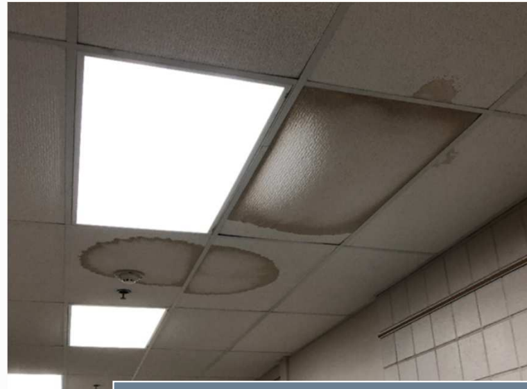
There are many damaged 2x4 ceiling tiles throughout facility due to roofing projects
