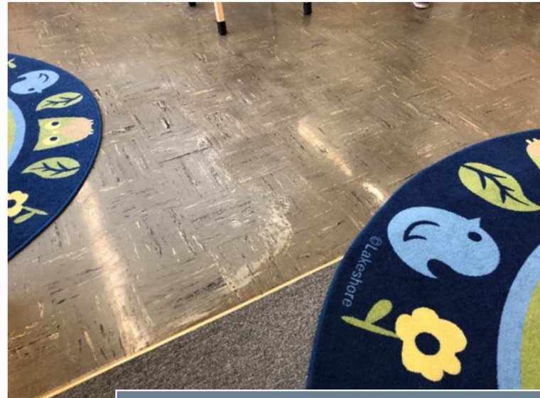
Asbestos containing flooring remaining in multiple classrooms
