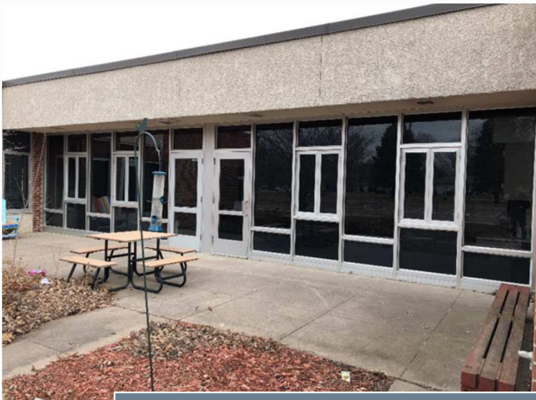
Original 1970 windows and doors need replacement
