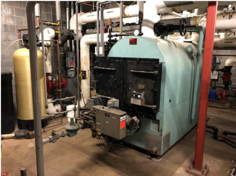
Hot water boilers and distribution systems
