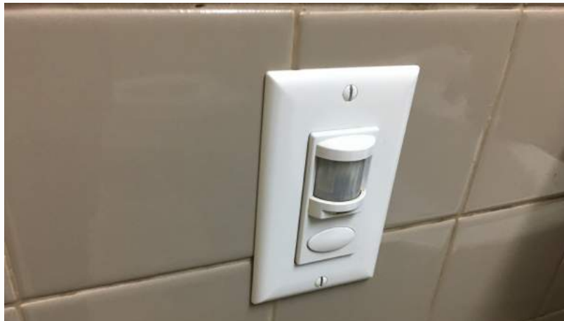
Occupancy controls installed with the LED lighting retrofit...
