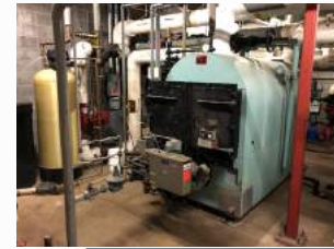
Hot water boilers and distribution systems
