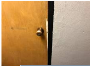
Many interior doors are older and have non-ADA compliant hardware
