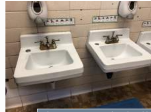
The restrooms are dated and have many older plumbing fixtures, tilework and toilet stall partitions
