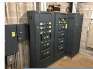
The main electrical service and distribution is original
