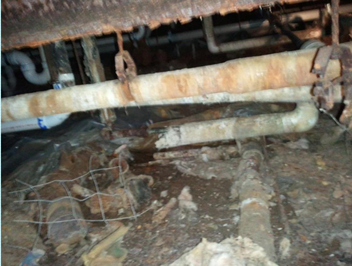
Sanitary pipes beneath Sterling
