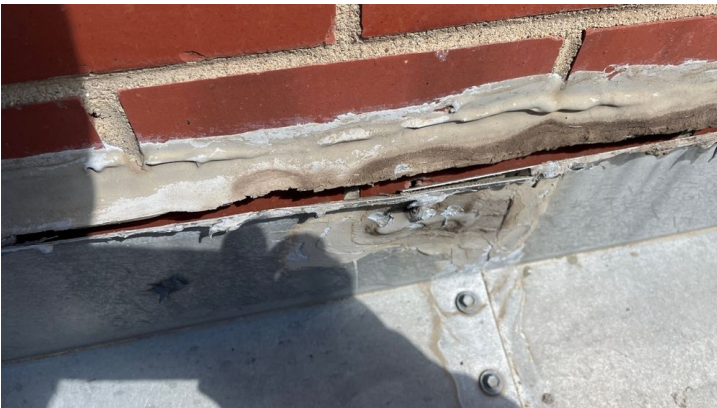
Photo showing missing wall fastener causing the wall counter flashings to back out.
