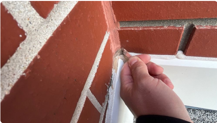
Photo showing silicone caulking failing in inside corner of the wall counter flashing.
