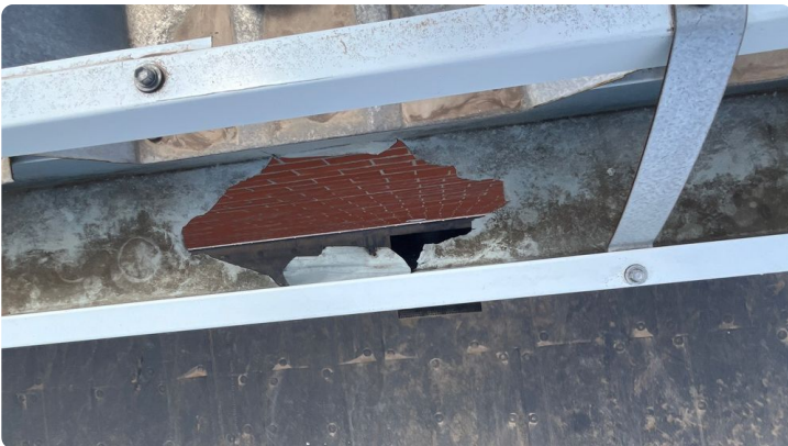
Photo showing hole in the gutter where the downspout detached.
