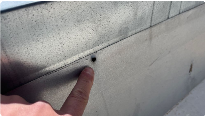
Photo showing a hole in the old covered skylights.
