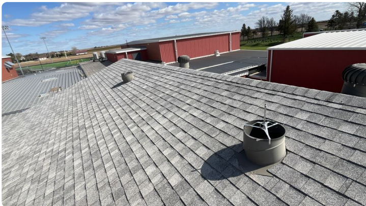
Photo showing two missing turbine caps.
