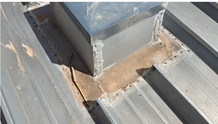
Photo showing sealant used throughout roof that is deteriorating around seams and flashings.
