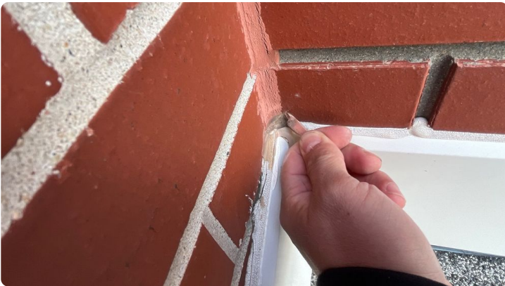
Photo showing silicone caulking failing in inside corner of the wall counter flashing.
