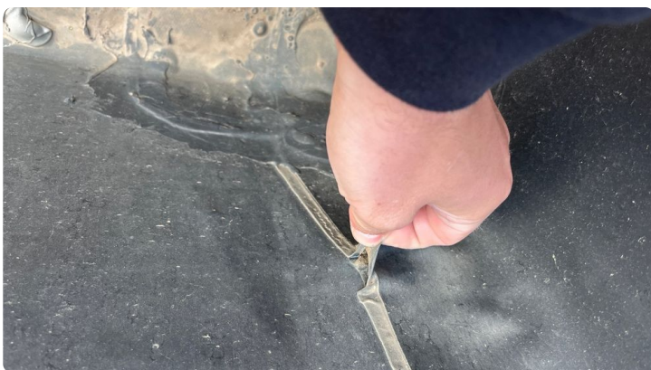
Photo showing an open wrinkle in the inside corner flashings causing a leak.
