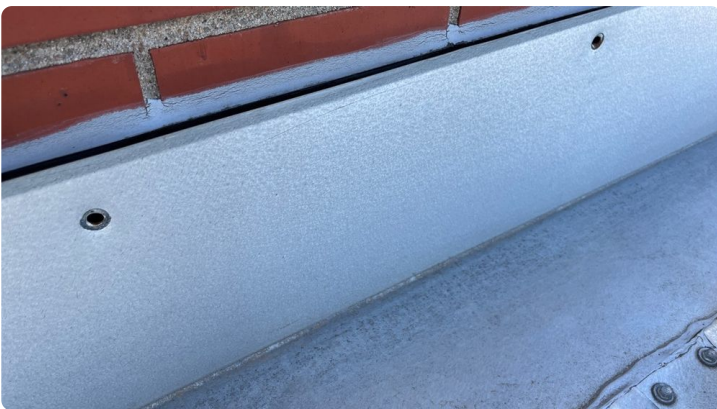
Photo showing missing chimney flashings fasteners.
