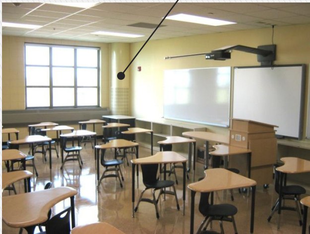
Displacement diffuser at corners
