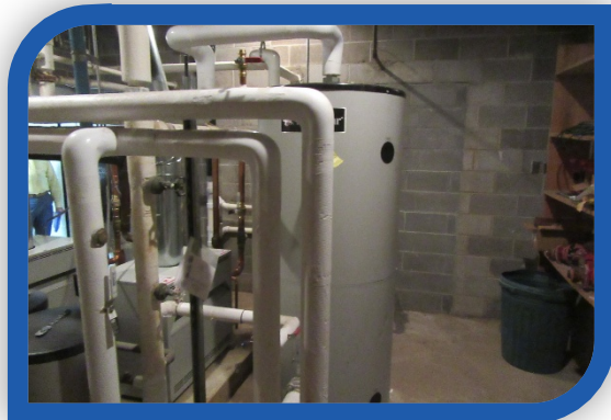
Domestic Hot Water Heater
