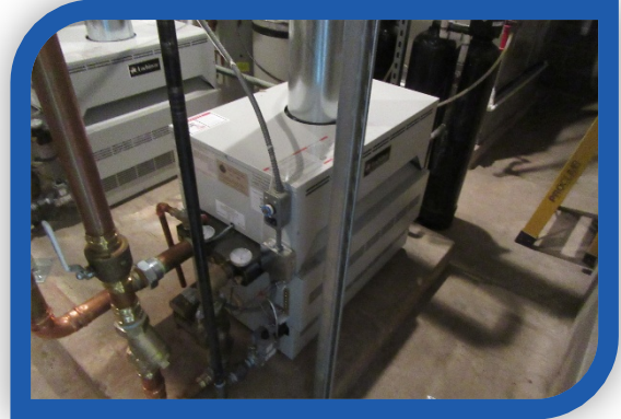
Hot Water Boiler
