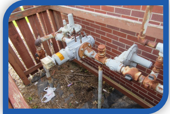
Natural Gas Meter
