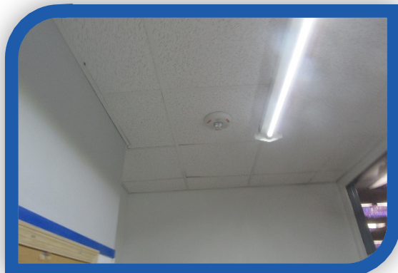
Fire Alarm Bell & Strobe
