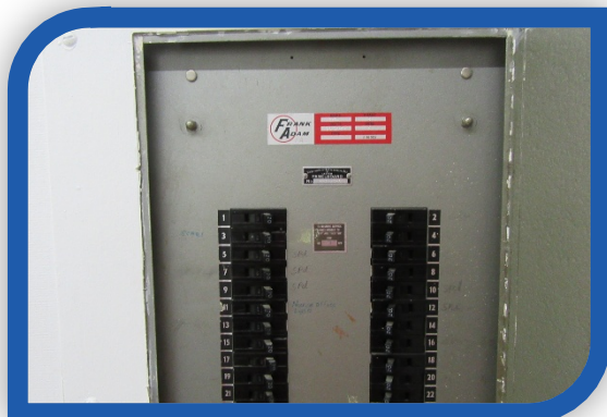
Obsolete Electrical Panel
