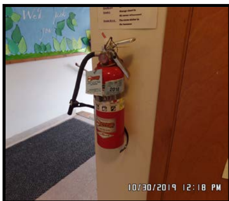
Out-dated inspection fire extinguisher Fisher School
