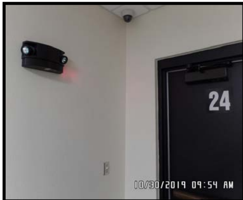
Door #24 emergency light non-operational High School
