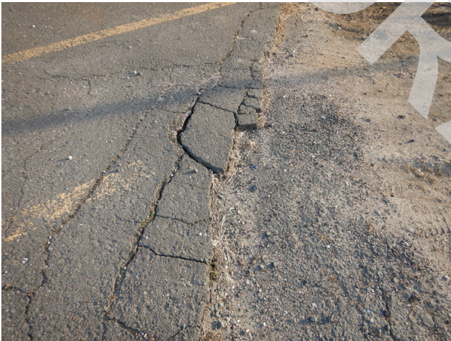
Asphalt vehicular pavement damage.
