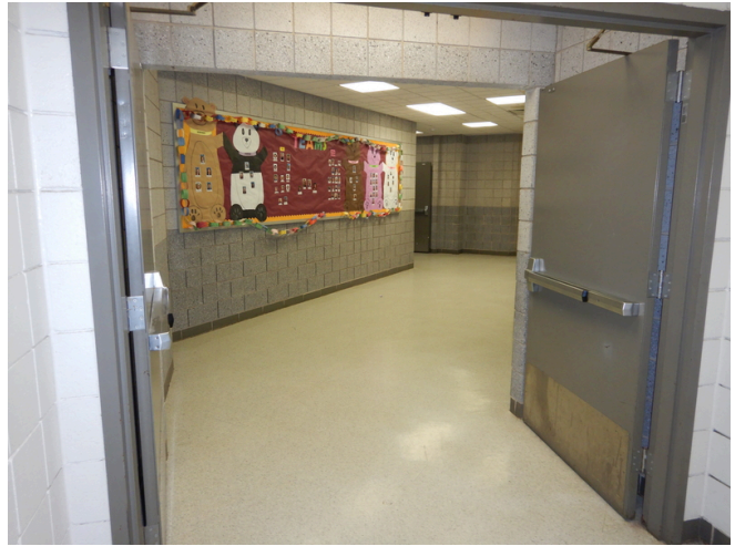
Corridor fire doors.
