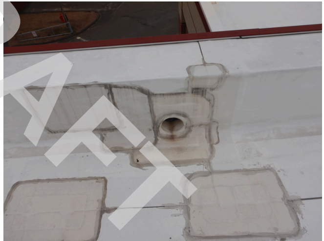
Gym: Evidence of TPO membrane repair.
