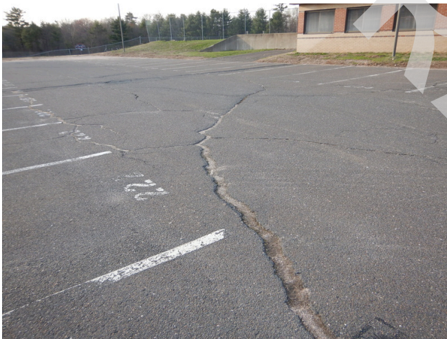
Linear cracking at the parking lot.
