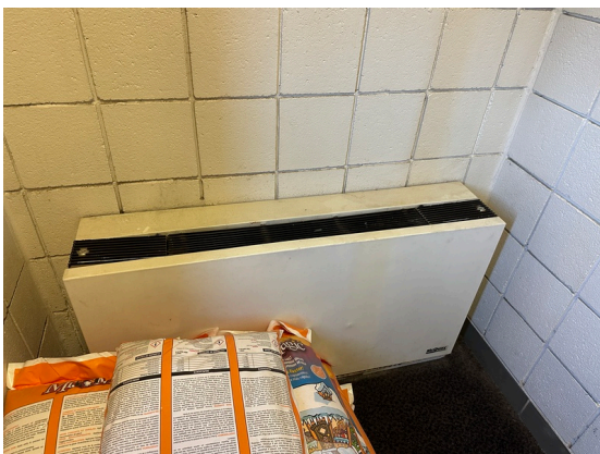
Photo 167: Typical HHW unit heater for stairwell.
