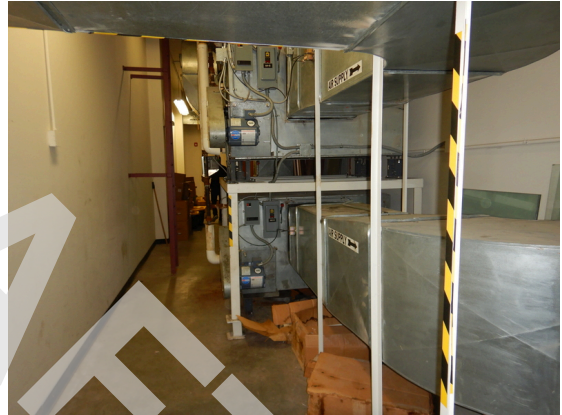
Photo 148: Second floor mechanical room.
