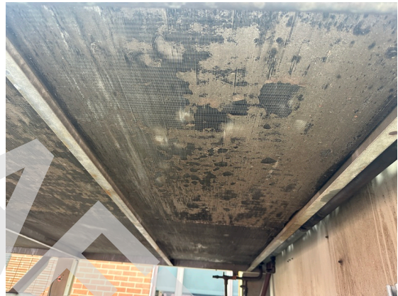
Photo 160: Typical condition of condensing unit fins.
