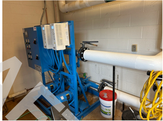
Photo 184: BLPs and controls cabinet.
