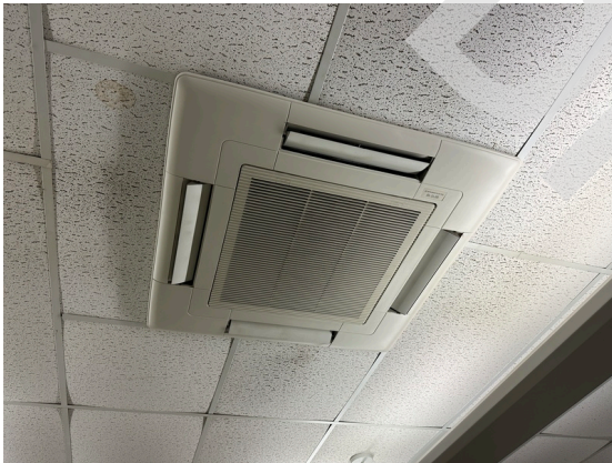
Photo 165: DX mini-split-system cassette unit.
