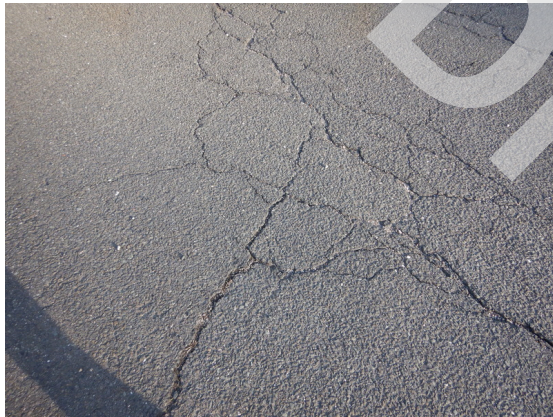
Photo 9: Typical alligator type cracking at the asphalt parking lot.
