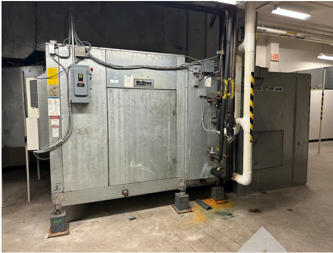
Typical Interior AHU with heating and cooling coils.
