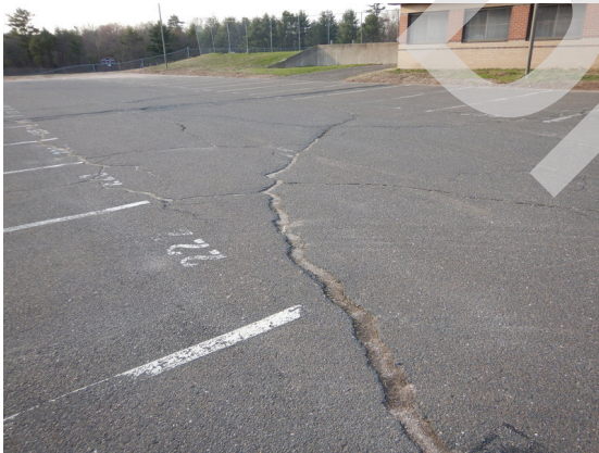
Photo 15: Linear cracking at the parking lot.
