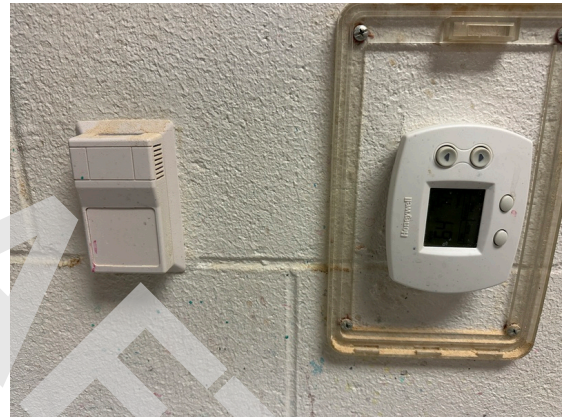
Photo 166: Typical older thermostat and temperature sensor.
