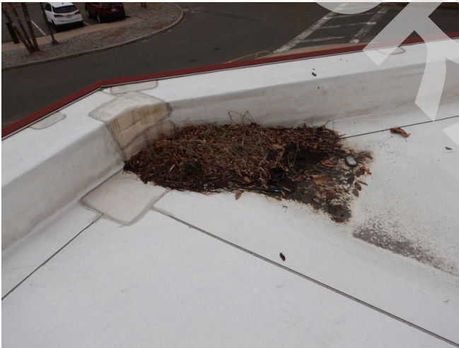
Ponding at the gym TPO membrane.
