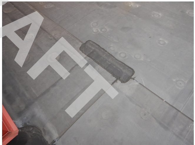
Evidence of previous repair of the EPDM roof membrane.
