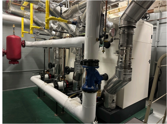
Photo 158: Typical condensing water boilers.
