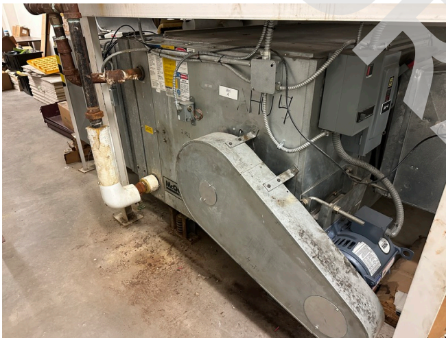
Typical AHU with heating coils only.
