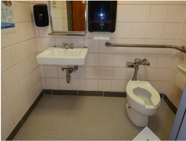
Clinic restroom toilet. Clinic r
