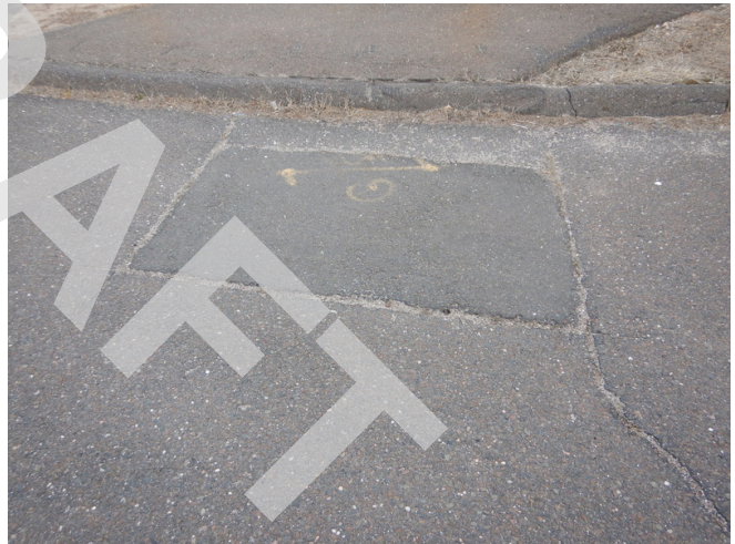
Evidence of previous repairs of asphalt vehicular pavement.
