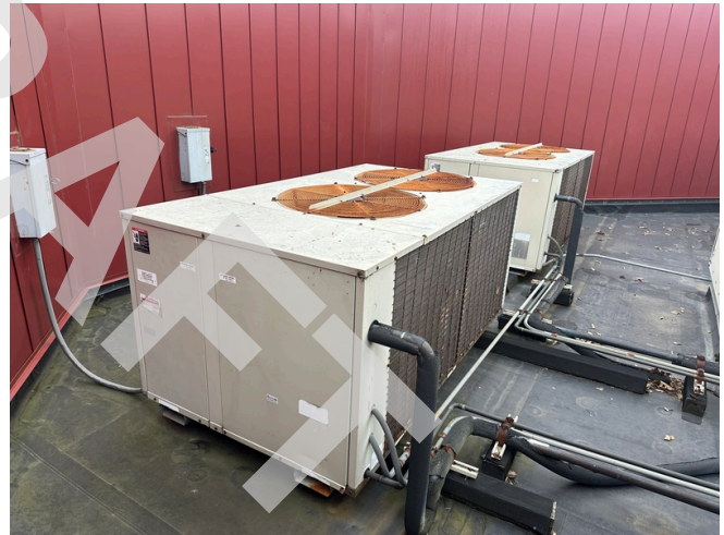
Typical roof-mounted condensing unit. Note corroded fan guards.
