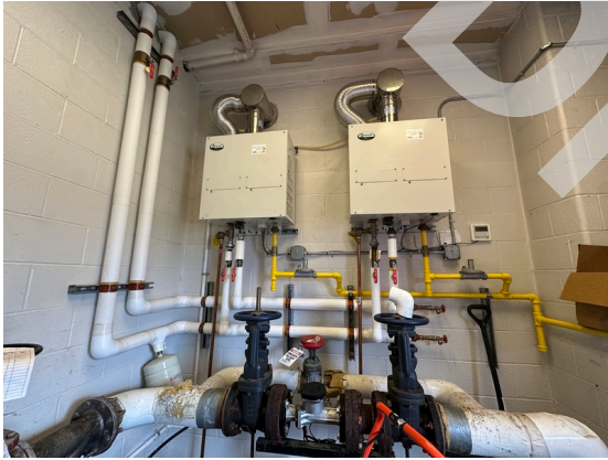
Photo 183: Tankless water heaters and domestic water backflow preventer.
