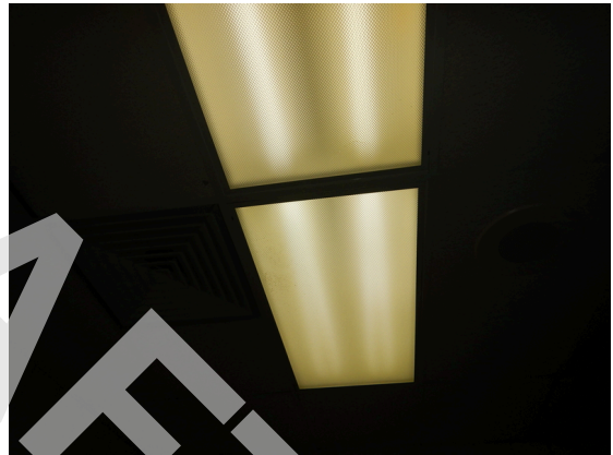
Photo 106: Typical florescent ceiling lighting.
