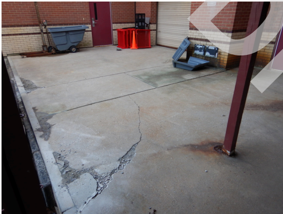
Photo 21: Damaged concrete pavement at the loading dock area. Typical of concrete pavement damage throughout.
