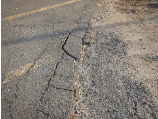
Photo 19: Asphalt vehicular pavement damage.
