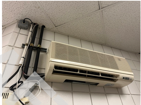
Photo 172: DX mini-split fan coil unit.
