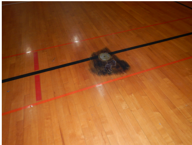
Gymnasium wood floor. Note the damaged spot.
