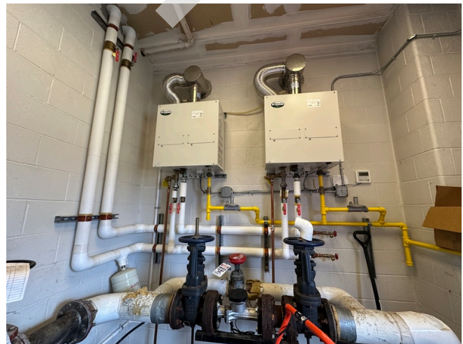
Tankless water heaters and domestic water backflow preventer.
