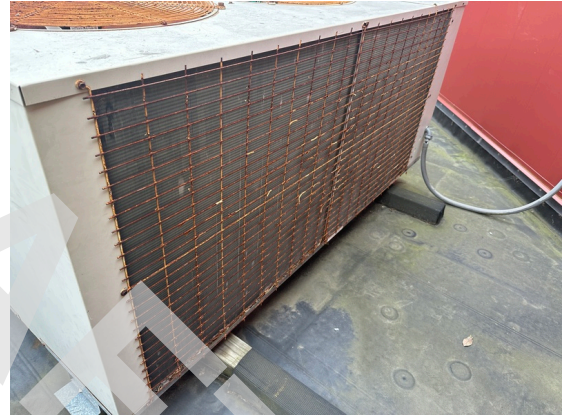
Photo 154: Typical condition of hail guards for condensing units. Note age and surface corrosion.
