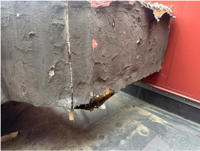
Typical condition of exterior ductwork, note deterioration of external coating/insulation.
