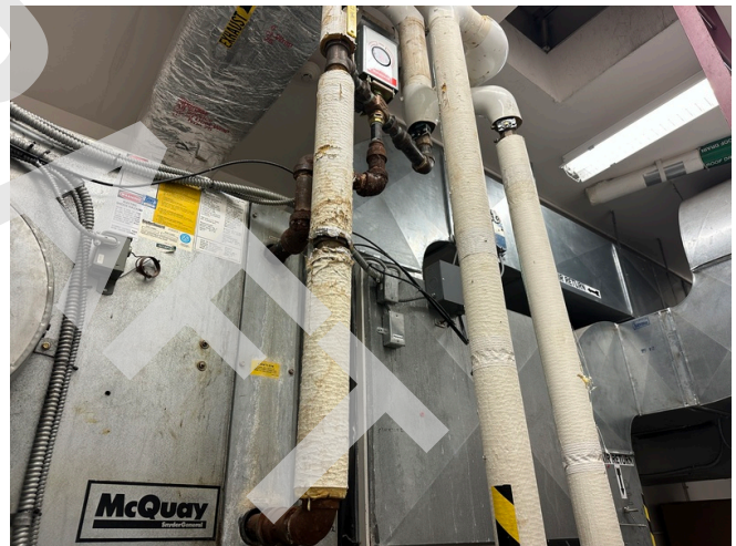
Typical condition of HHW piping, connections, and insulation.
