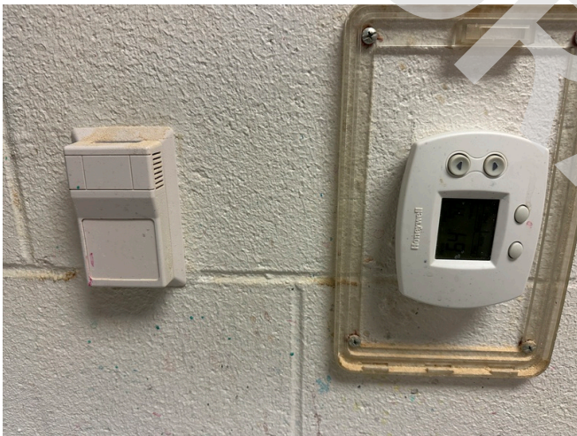
Typical older thermostat and temperature sensor.
