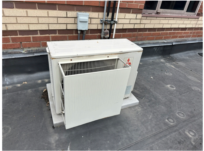
DX mini-split condensing unit.
