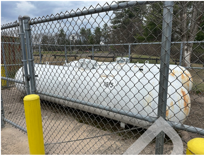
Chain link fence surrounding propane tanks for kitchen equipment.
