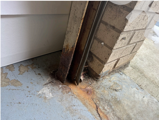
Corrosion on base of roll-up door in maintenance room.
