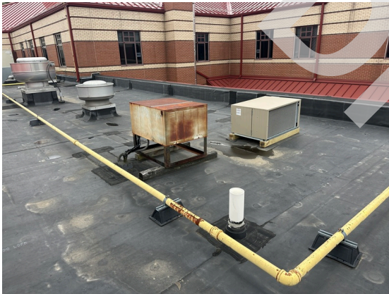
Photo 159: Typical roof-mounted equipment. Note surface corrosion on natural gas piping.
