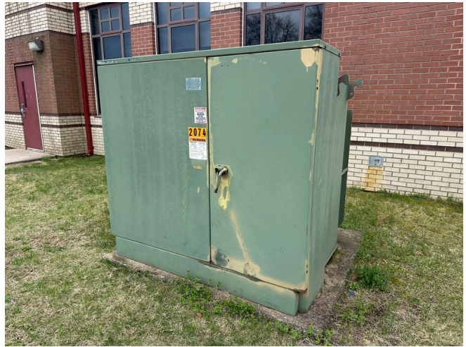
Utility owned, pad-mounted transformer.
