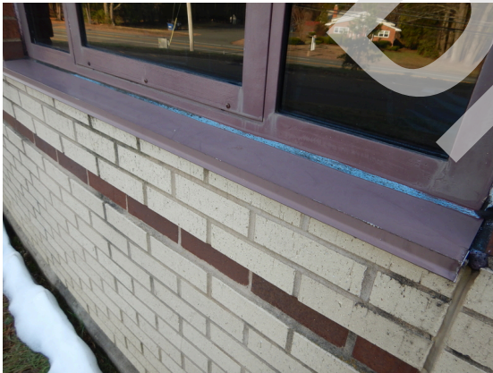
Photo 45: Brick veneer bellow windows.
