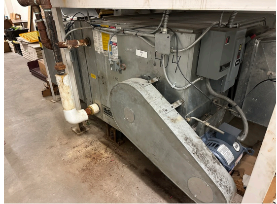
Photo 170: Typical AHU with heating coils only.
