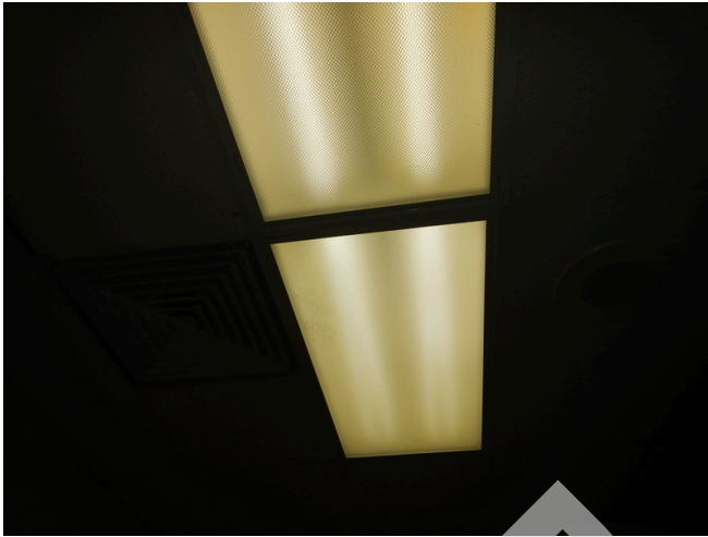
Typical florescent ceiling lighting.
