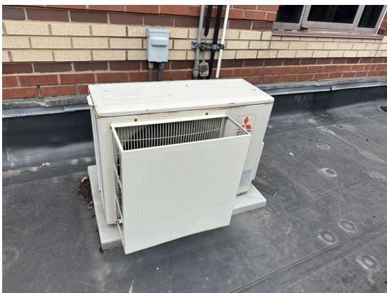
Photo 161: DX mini-split condensing unit.
