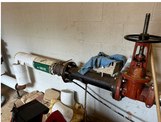
Photo 191: Fire suppression backflow preventer.
