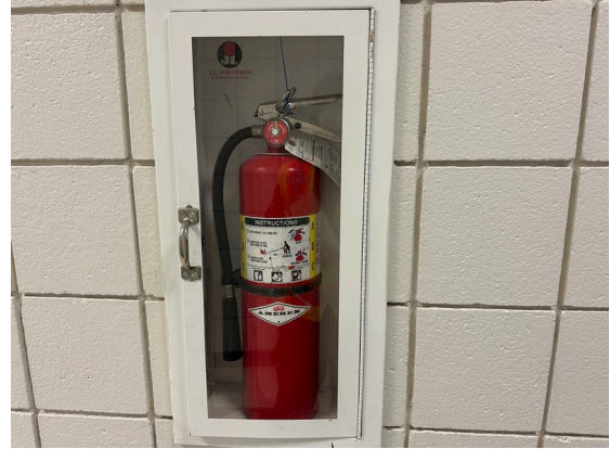
Photo 188: Typical portable fire extinguisher in cabinet.
