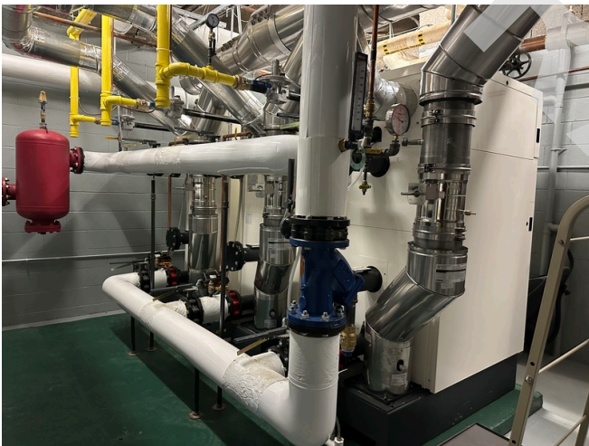
Typical condensing water boilers.
