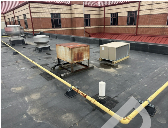
Typical roof-mounted equipment. Note surface corrosion on natural gas piping.
