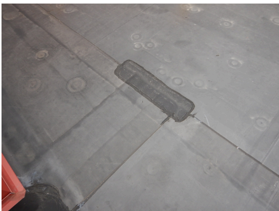
Photo 53: Evidence of previous repair of the EPDM roof membrane.
