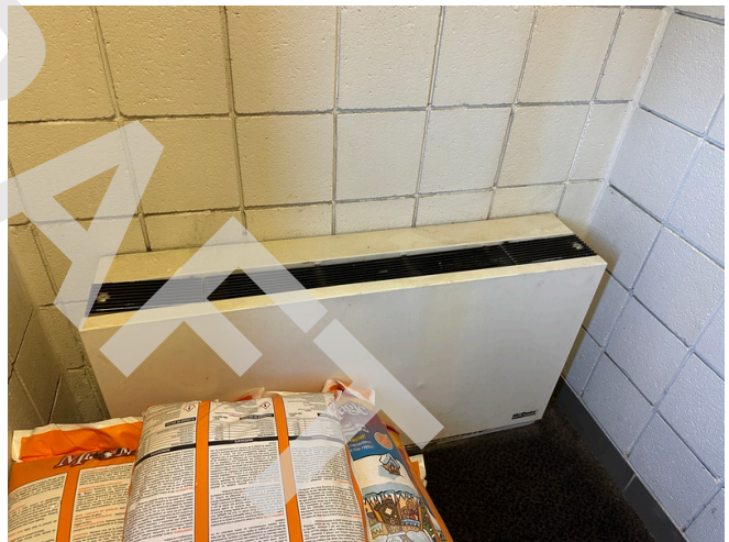
Typical HHW unit heater for stairwell.
