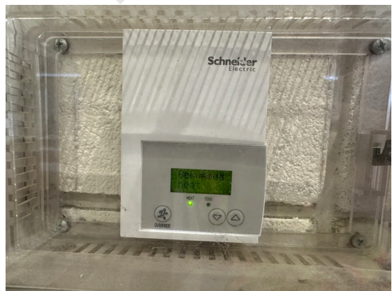
Photo 162: Typical new wall-mounted thermostat.
