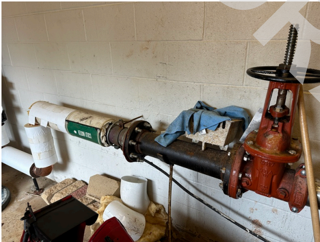
Fire suppression backflow preventer.
