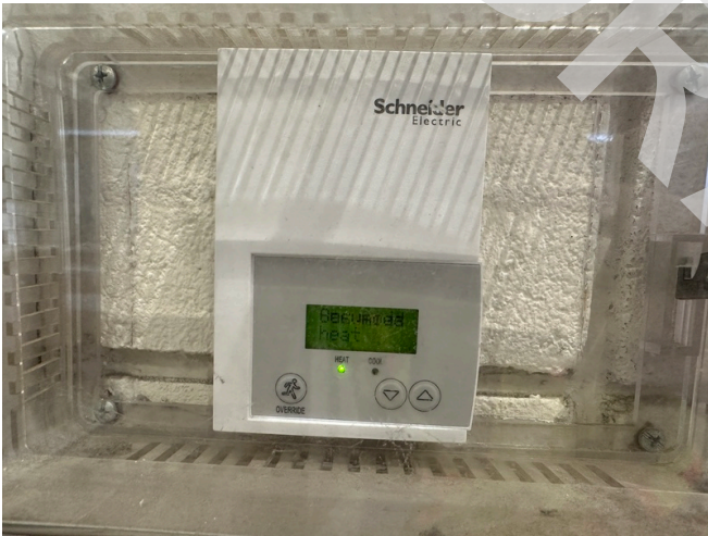
Typical new wall-mounted thermostat.
