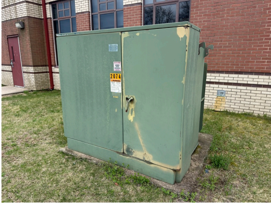
Photo 181: Utility owned, pad-mounted transformer.
