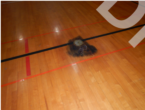
Photo 27: Gymnasium wood floor. Note the damaged spot.
