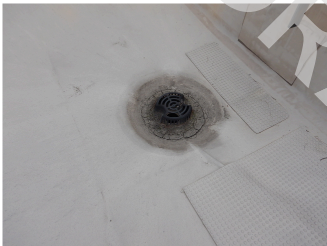
Gym: internal drain.
