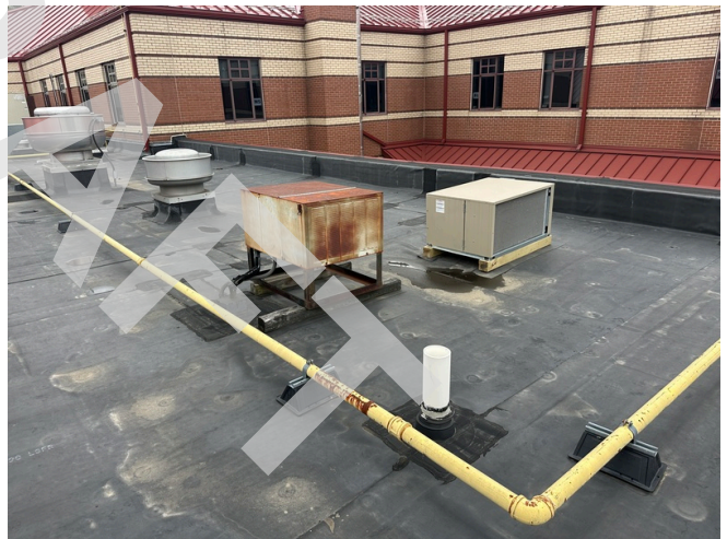
Typical roof-mounted equipment. Note surface corrosion on natural gas piping.
