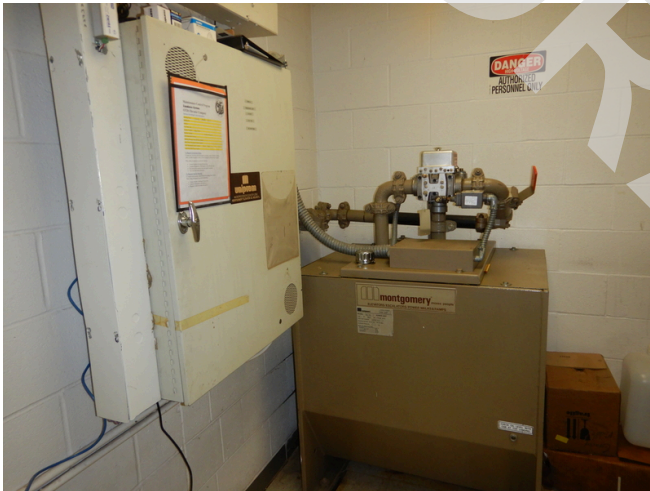
Elevator equipment room.
