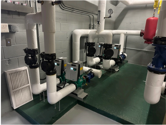
Photo 157: HHW Circulation pumps.
