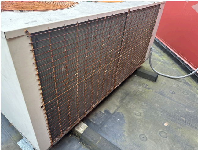
Typical condition of hail guards for condensing units. Note age and surface corrosion.
