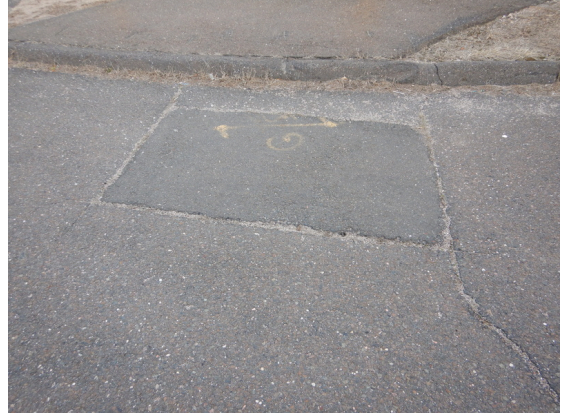
Photo 20: Evidence of previous repairs of asphalt vehicular pavement.
