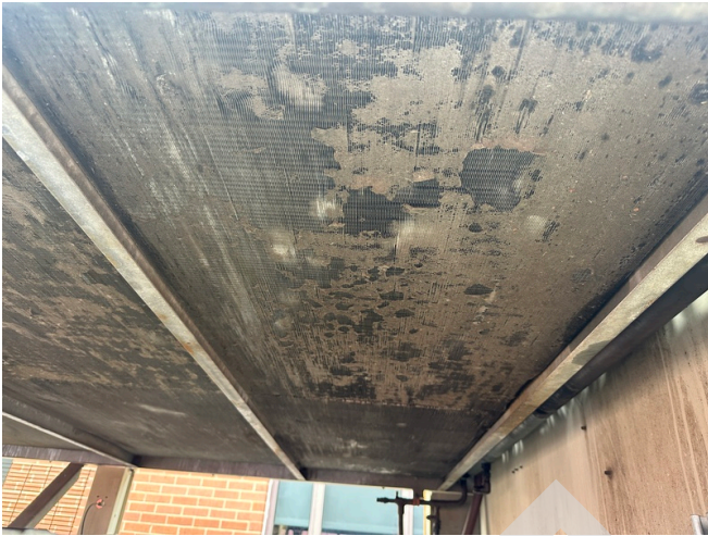
Typical condition of condensing unit fins.
