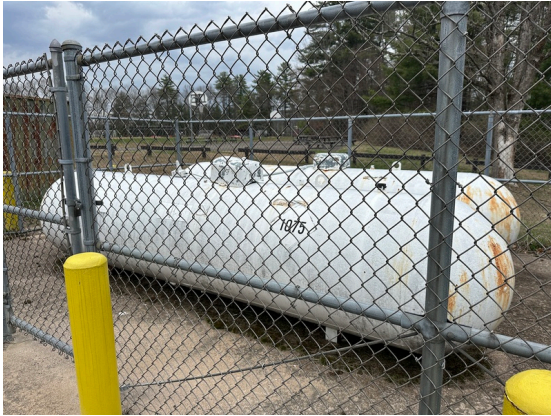
Photo 1: Chain link fence surrounding propane tanks for kitchen equipment.
