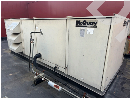
Photo 177: Typical roof-mounted AHU with heating and cooling coils.
