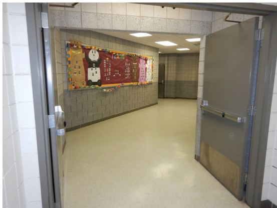
Photo 107: Corridor fire doors.
