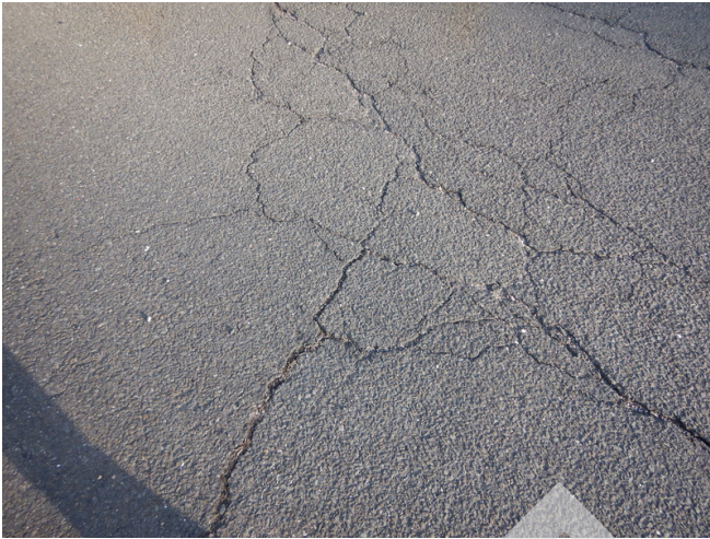
Typical alligator type cracking at the asphalt parking lot.
