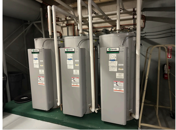
Photo 182: Tank-type water heaters.
