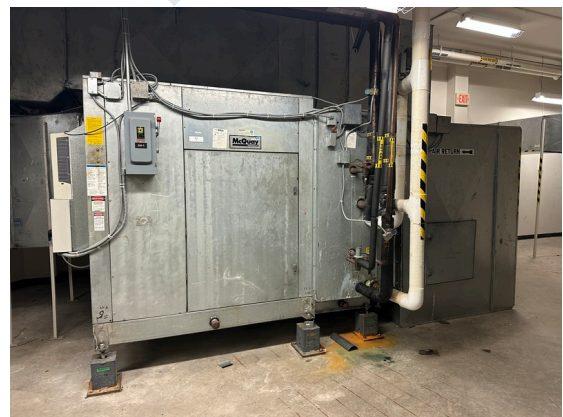
Photo 168: Typical Interior AHU with heating and cooling coils.
