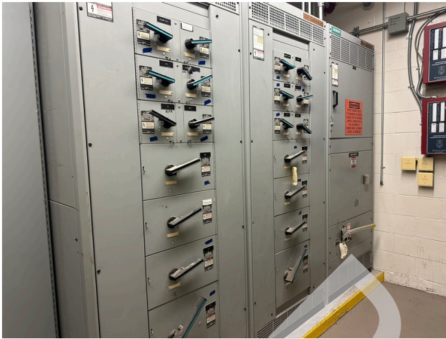
Main Electrical Switchboard.
