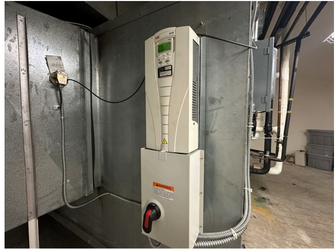
Typical VFD for interior AHU.
