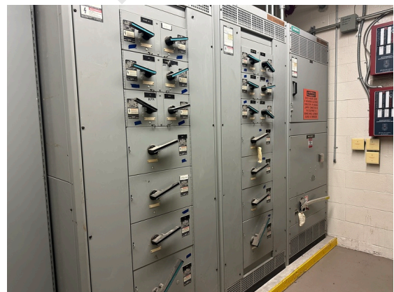
Photo 180: Main Electrical Switchboard.
