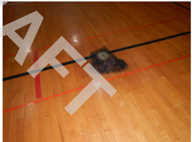
Gymnasium wood floor. Note the damaged spot.
