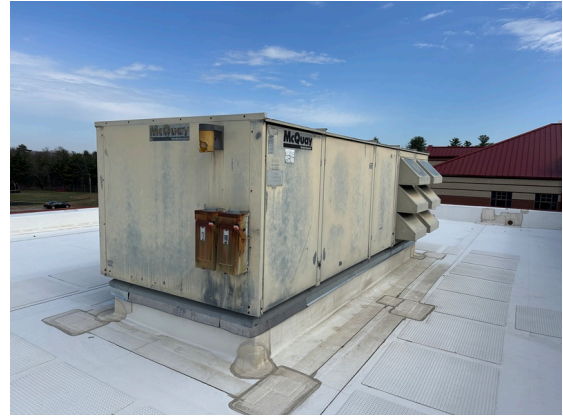
Photo 164: Typical roof-mounted VAV-AHU with heating only.
