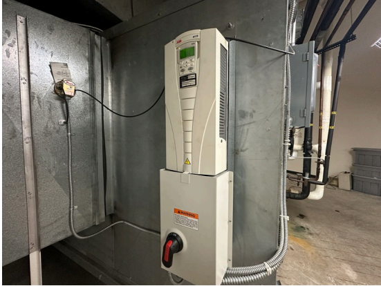
Photo 169: Typical VFD for interior AHU.
