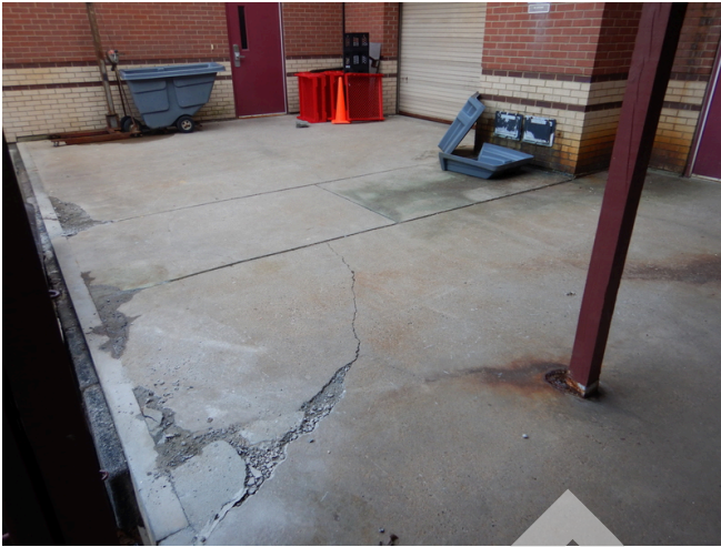
Damaged concrete pavement at the loading dock area. Typical of concrete pavement damage throughout.
