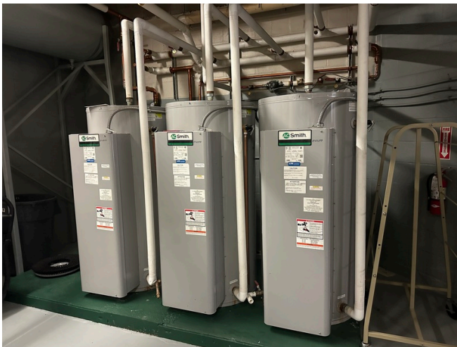
Tank-type water heaters.
