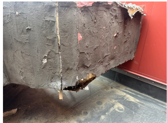
Photo 156: Typical condition of exterior ductwork, note deterioration of external coating/insulation.
