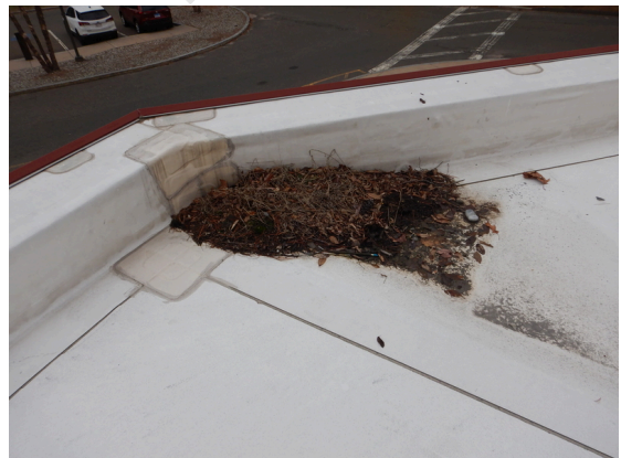
Photo 60: Ponding at the gym TPO membrane.
