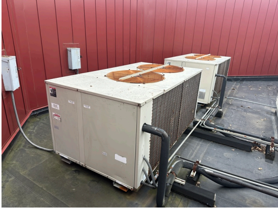
Photo 175: Typical roof-mounted condensing unit. Note corroded fan guards.
