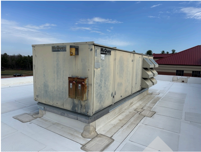
Typical roof-mounted VAV-AHU with heating only.
