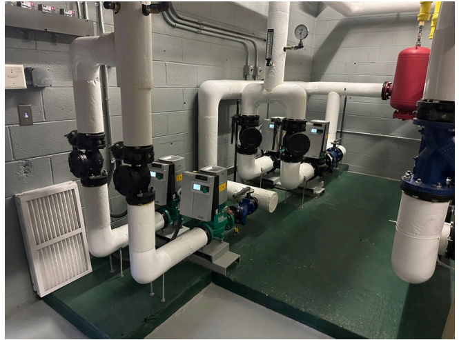
HHW Circulation pumps.
