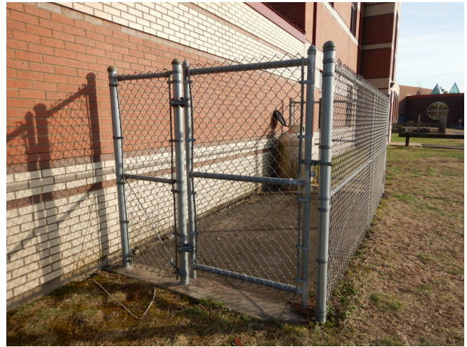
Chain link fence surrounding propane tank at the loading dock area.
