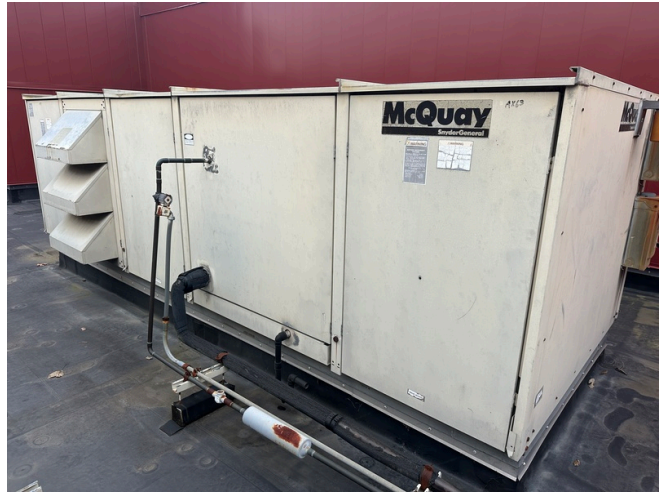
Typical roof-mounted AHU with heating and cooling coils.
