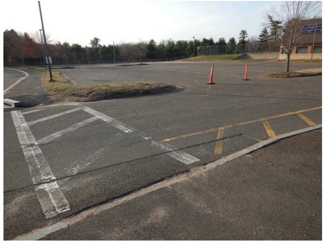
Overview of the main parking lot at the rear of the building.
