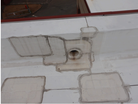
Photo 61: Gym: Evidence of TPO membrane repair.
