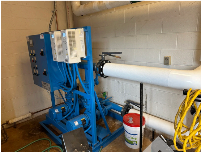
BLPs and controls cabinet.
