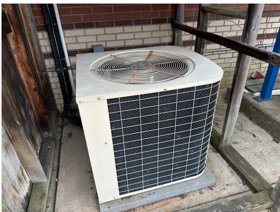
Photo 173: DX split-system condensing unit.
