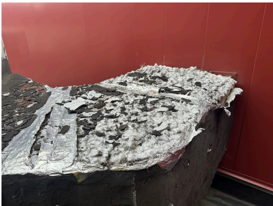
Photo 155: Typical condition of exterior ductwork.
