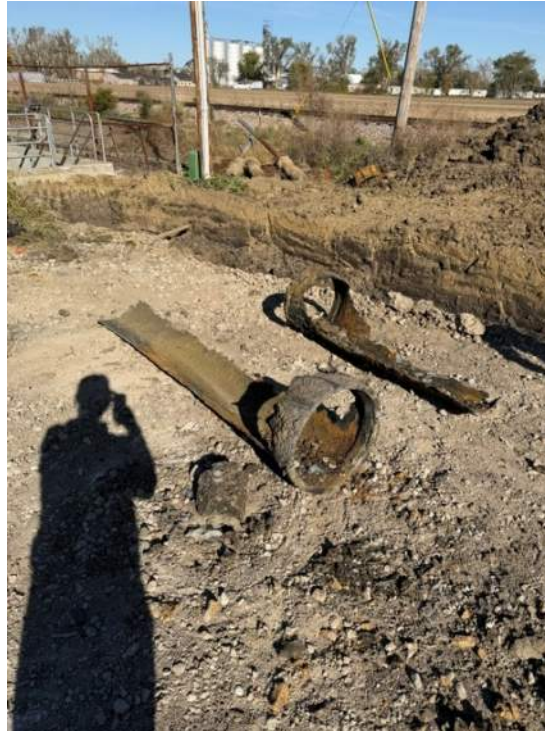
Figure 2-3. Previous Ductile Iron Pipe Sections that were Replaced
