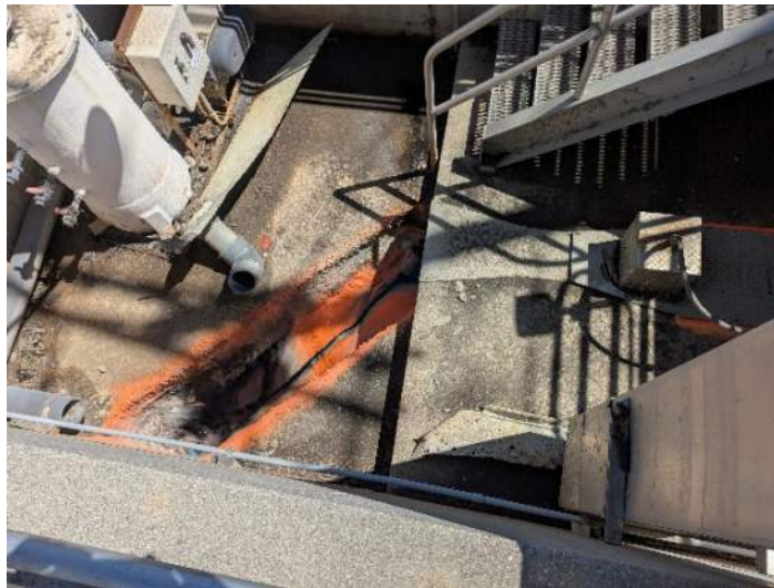
Figure 2-1. Existing Force Main Outfall and Non-Operational Carbon Scrubber
