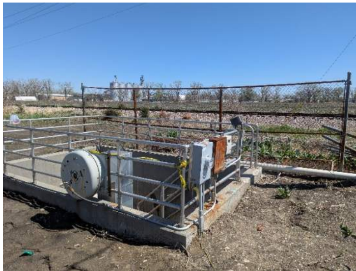
Figure 2-2. Existing Force Main Discharge Structure and Observed Corrosion
