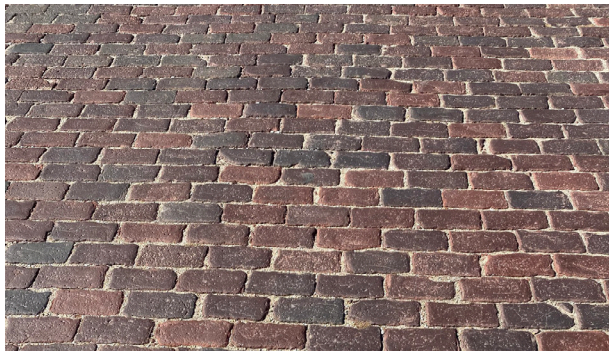
FIGURE 2.28 / BRICKS ON 1ST STREET HAVE SHIFTED OVER TIME
