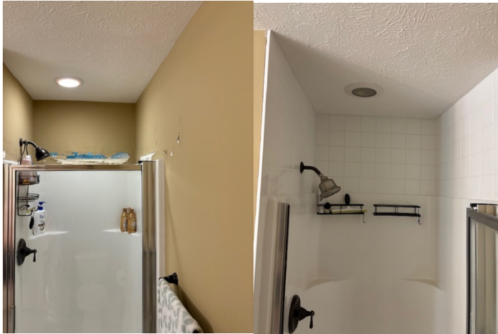
Completed shower tile project from Building & Construction class: Mr. Mattes, Luke Vitallo and Leora Hoffman.
