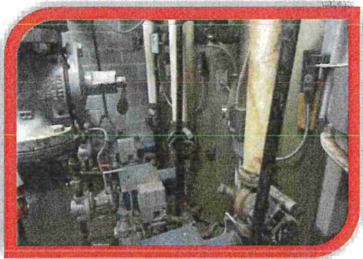
Hot Water Boiler System
