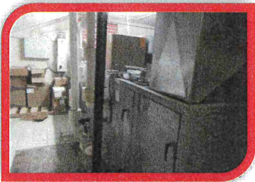
Air Handling Unit
