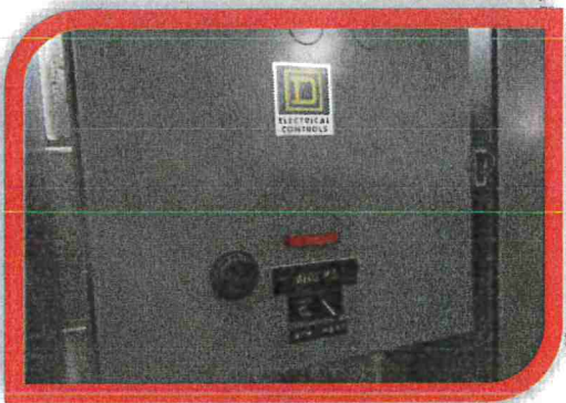
AHU Electrical Disconnect
