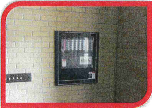
Fire Alarm System
