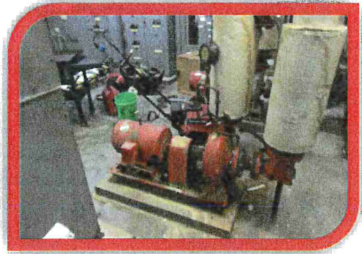
Hydronic Distribution Pumps
