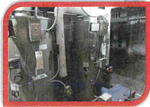
Hot Water Boilers
