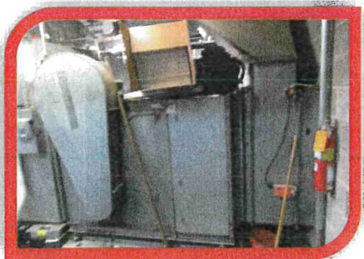
Air Handling Unit
