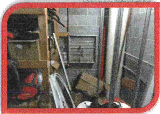
Outside Air Damper
