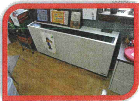
Unit Ventilator Terminal Unit
