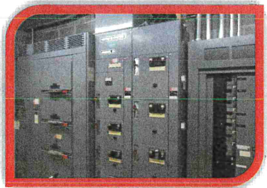
Electrical Distribution System
