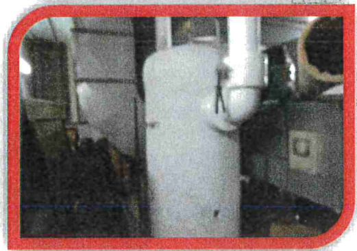
Air Handling Unit
