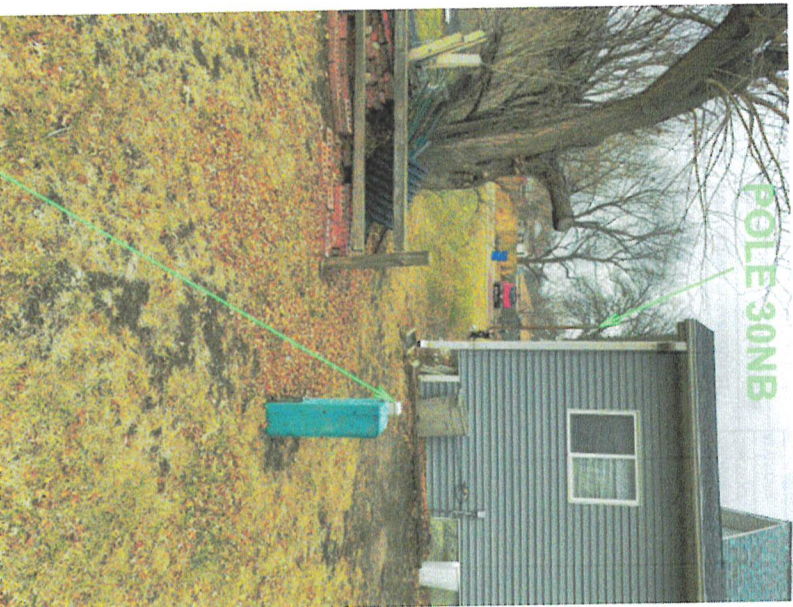
COPPER PED 35NB LOOKING NORTH
