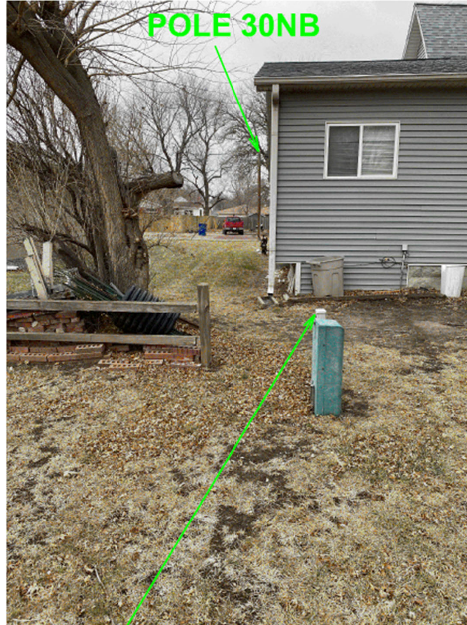
POLE 30NB COPPER PED 35NB LOOKING NORTH
