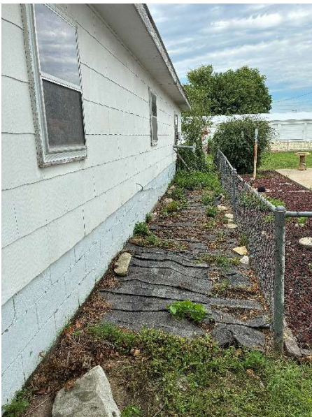
Figure S. Shingle placement and vegetation conditions in rear yard
