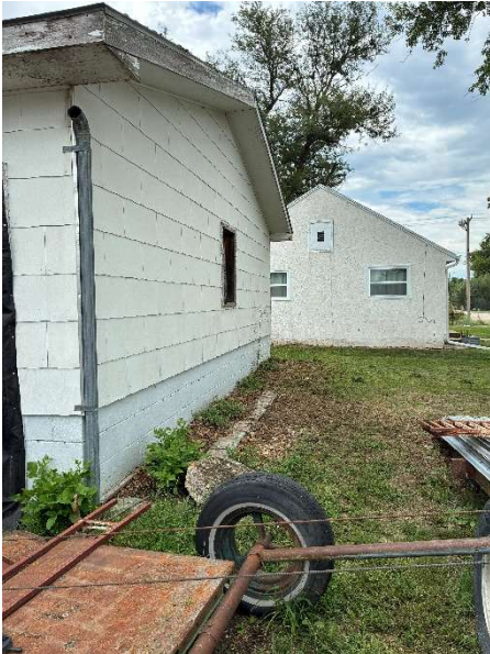
Figure U. Vegetation conditions in south side yard
