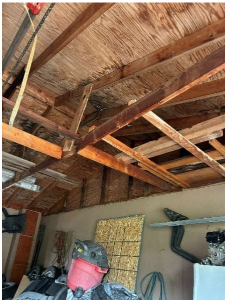
Figure G. Bowing support beam on south side of garage
