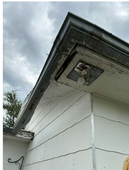
Figure L. Gutter system of garage and residence in disrepair
