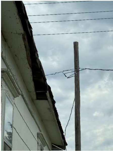
Figure E. Deteriorated soffit and fascia on north side of residence
