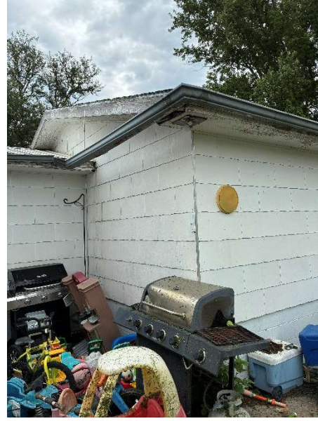
Figure J. Gutter system of residence and garage in disrepair
