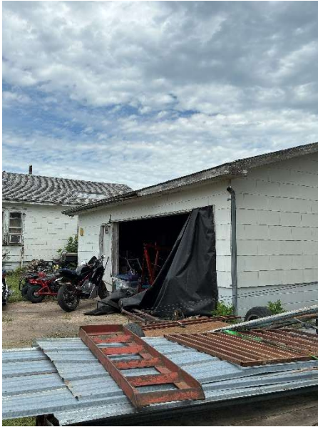
Figure A. Missing garage door with tarp being used as temporary cover
