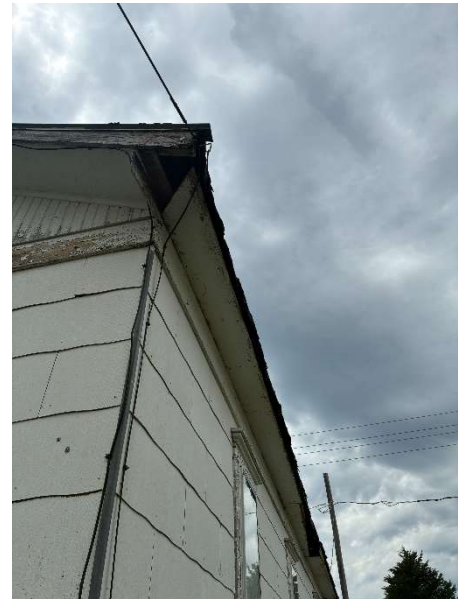
Figure F. Deteriorated soffit and fascia on north side of residence
