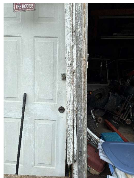
Figure P. Entry door of garage in disrepair and splitting at bottom
