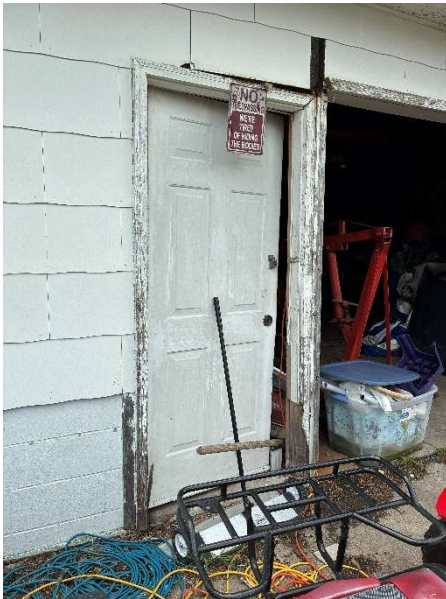
Figure M. Entry door of garage in disrepair
