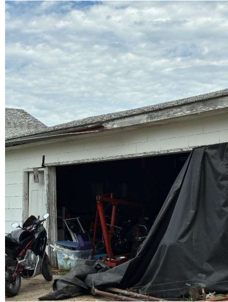
Figure B. Missing garage door and gutter system
