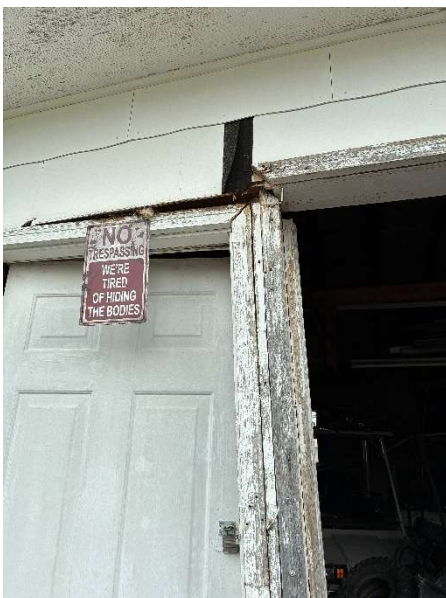
Figure O. Entry door of garage in disrepair and leaning on door frame
