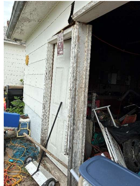
Figure N. Entry door of garage in disrepair
