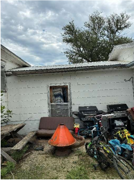
Figure I. Gutter system of residence in disrepair
