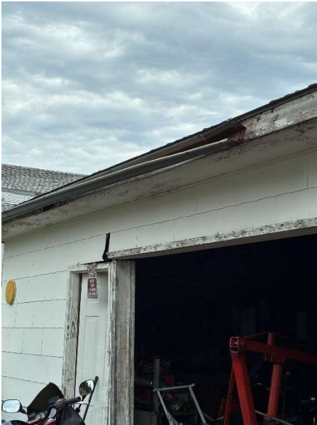
Figure K. Gutter system of garage in disrepair
