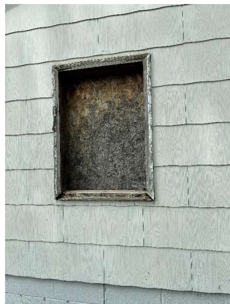
Figure D. Boarded up garage window
