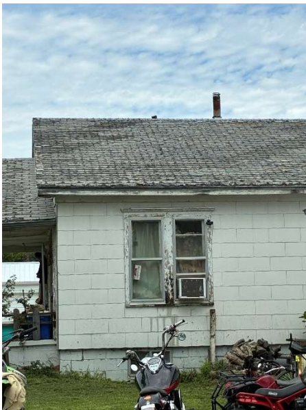
Figure C. Roof shingles of residence in disrepair
