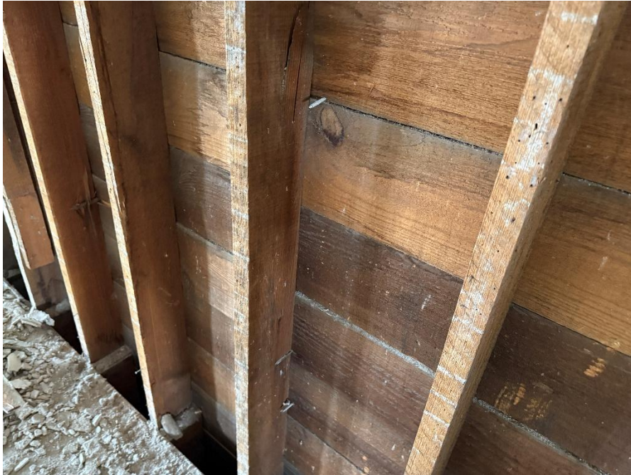
Photo 9 - Exposed lag screws at south wall.
