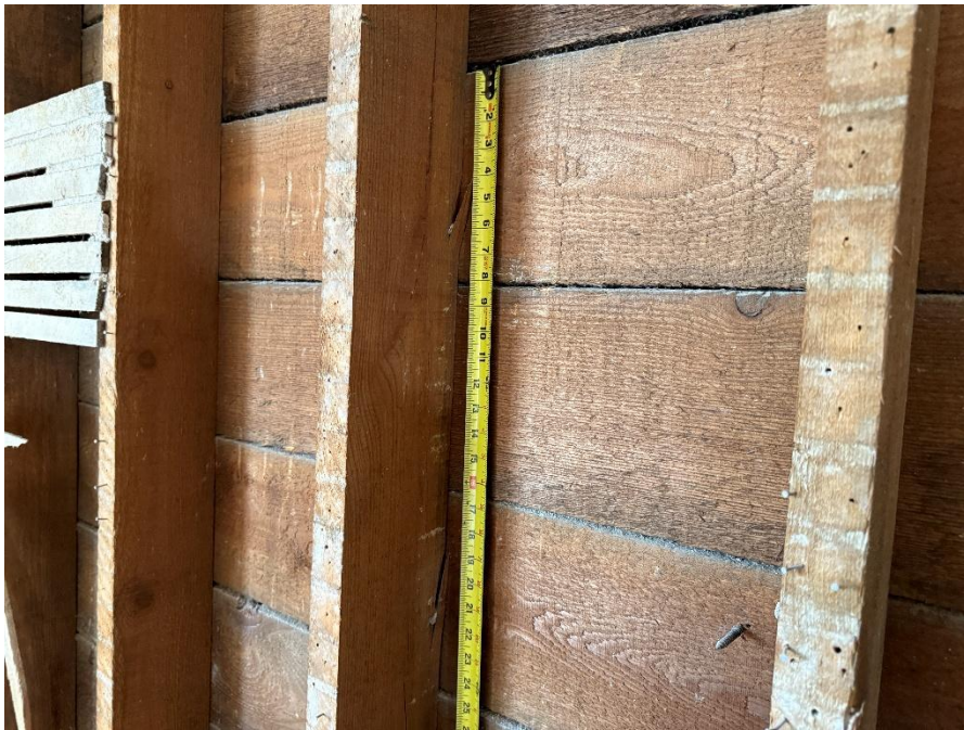
Photo 8 - Lag screws exposed at south wall.
