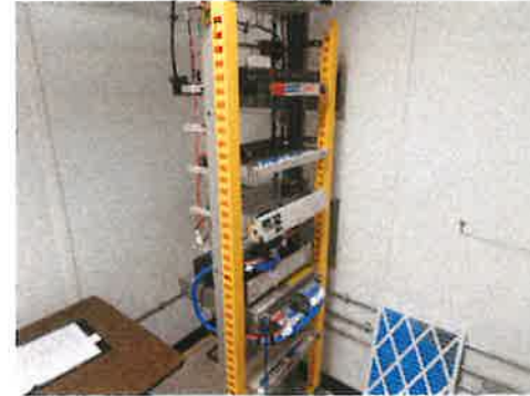
EQUIPMENT INSIDE SHELTER SCALE NTS
