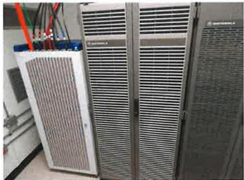
EQUIPMENT INSIDE SHELTER SCALE: NTS
