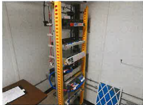
EQUIPMENT INSIDE SHELTER SCALE: NTS
