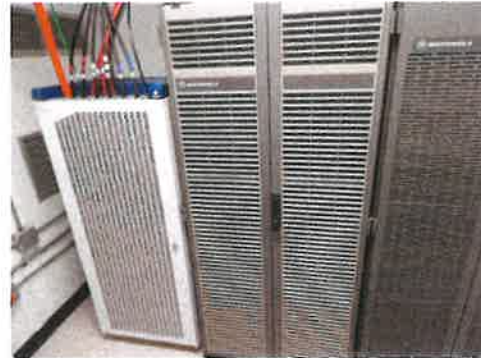
EQUIPMENT INSIDE SHELTER SCALE NTS
