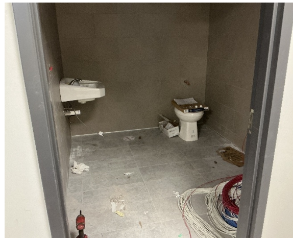
Plumbing finishes on the 1st floor
