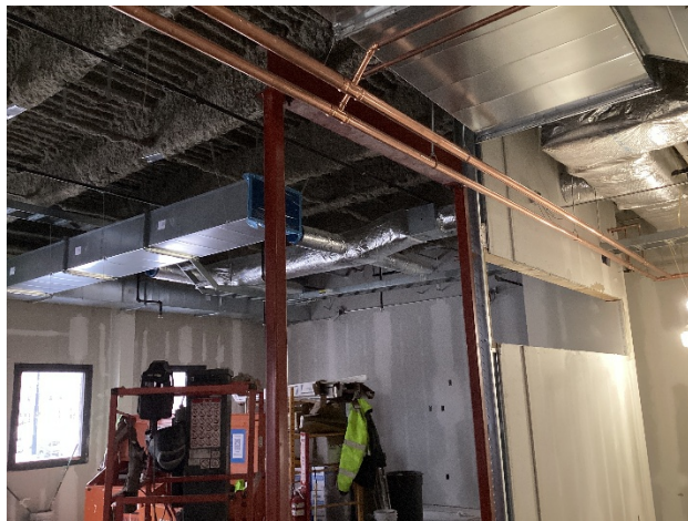
Mechanical Heating Lines
