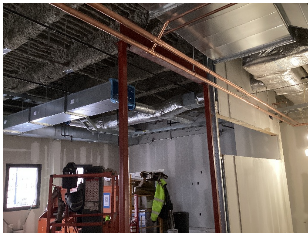
Mechanical Heating Lines
