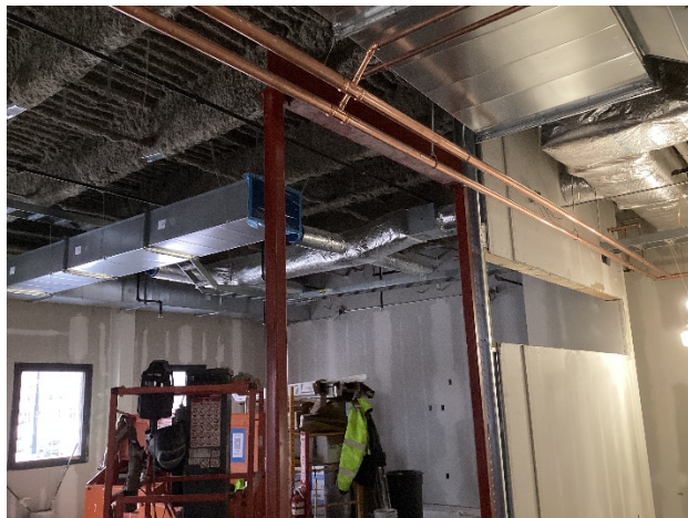
Mechanical Heating Lines
