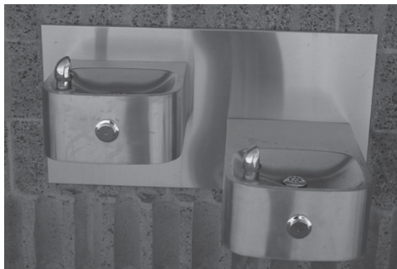
Fountains Connected to a Central Chiller
