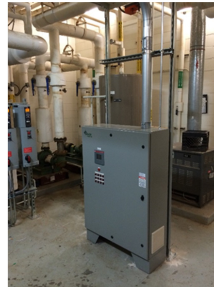
Installation of capacitor banks can correct PF to 95%
