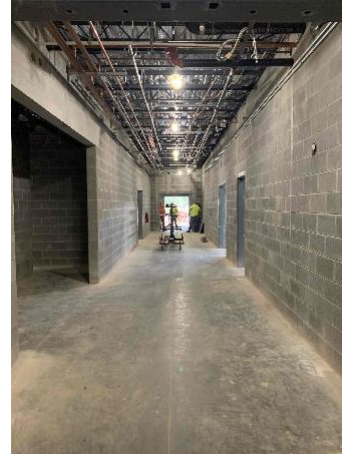
Gym Hallway - Above Ceiling - Mechanical Electrical and Plumbing
