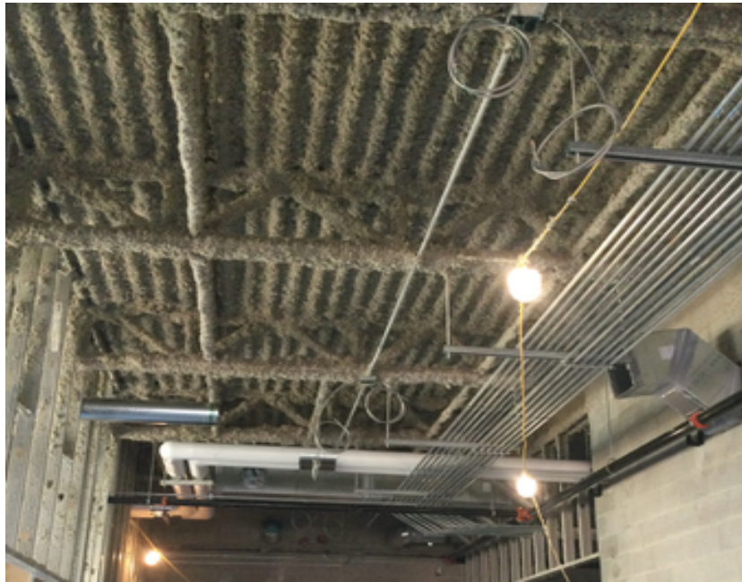
Above ceiling on third floor
