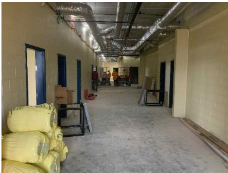
Overhead HVAC Duct on 2 nd Floor
