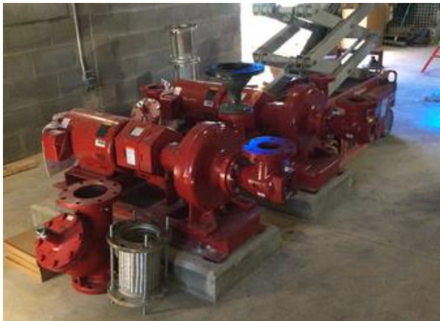
Geothermal circulation pumps
